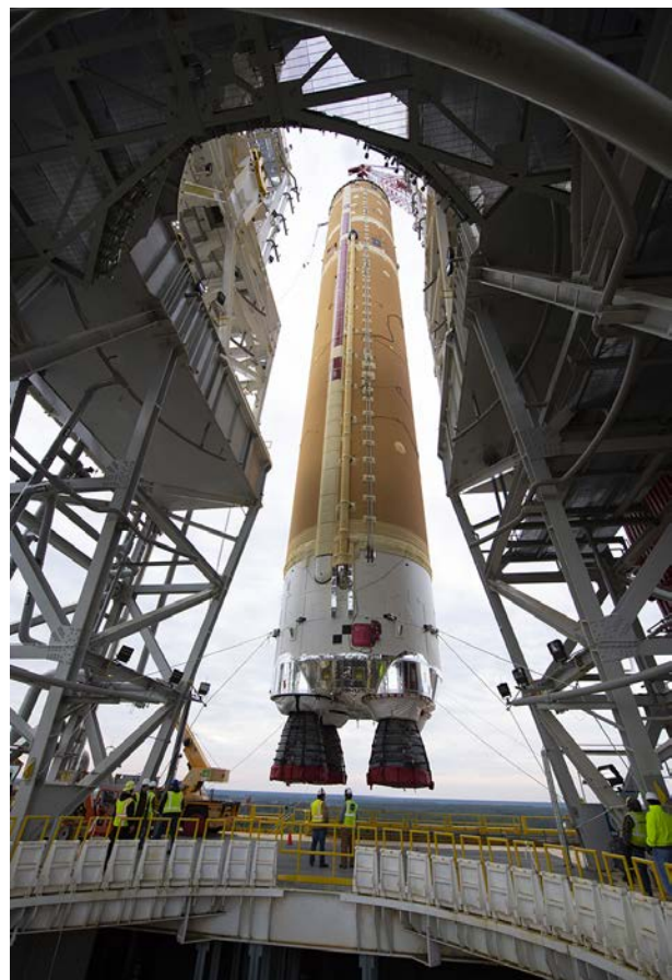
Crews at Stennis Space Center lift and install the first Core Stage of the SLS into the B-2 Test Stand
