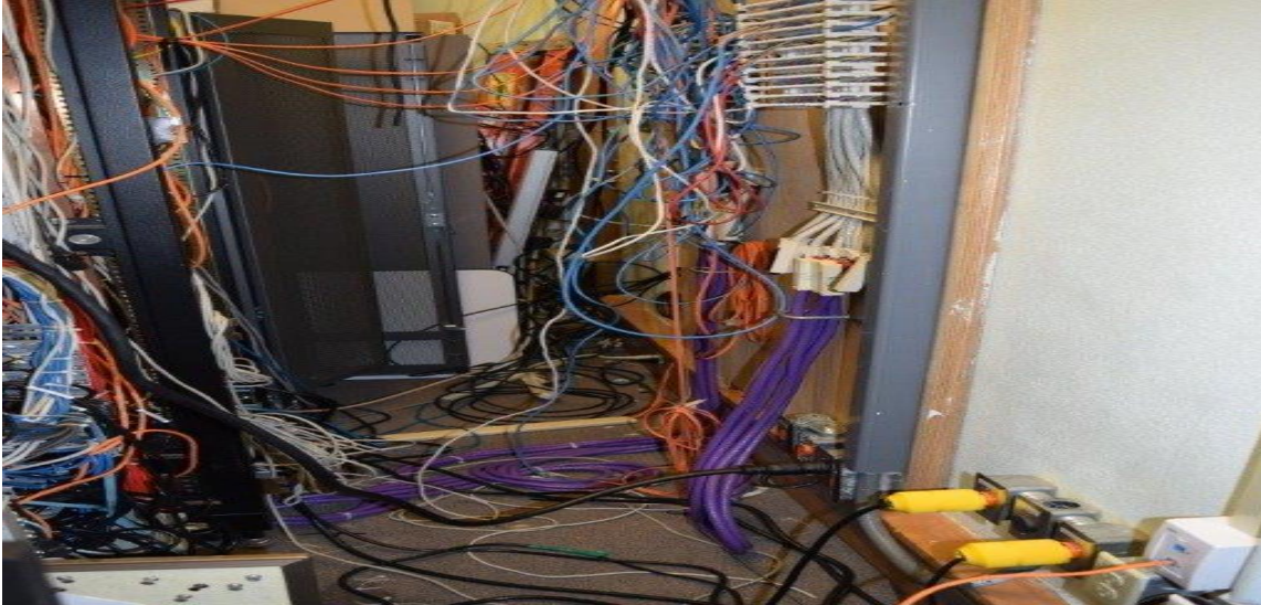
Figure 1: Embassy Georgetown Unclassified Server Room (Source: Embassy Georgetown)
