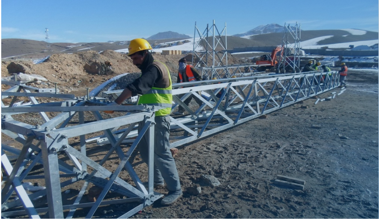
Workers install the equipment to erect an electricity tower linking Kabul to Kandahar and Helmand, Afghanistan. Photo: USAID/Afghanistan (Jan. 17, 2016)
