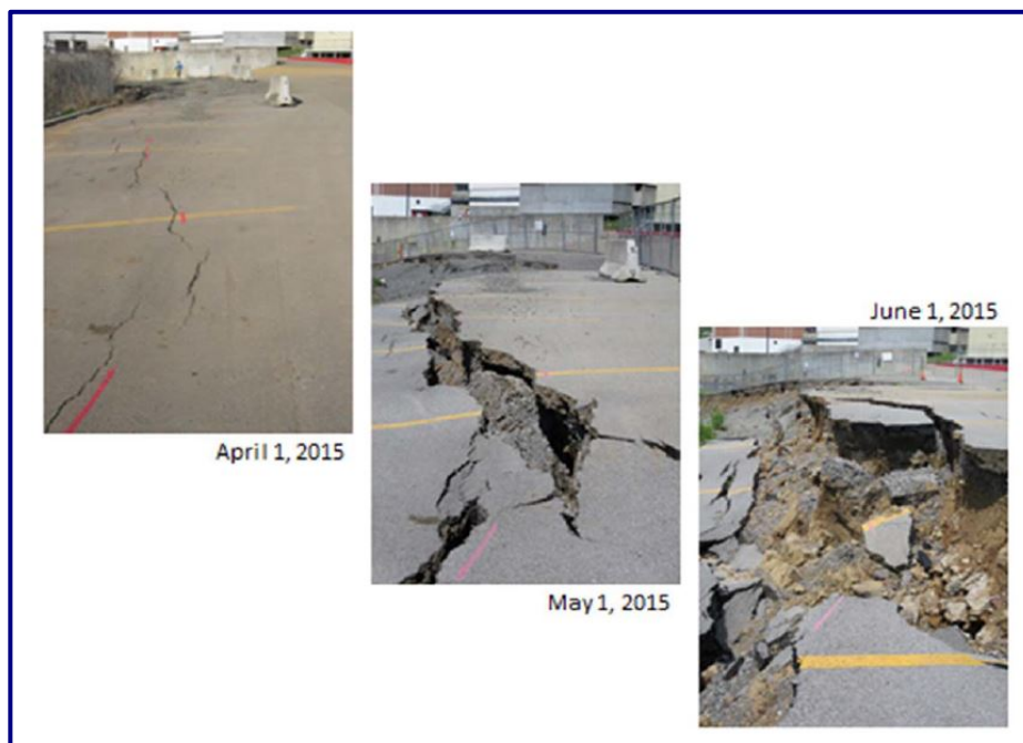
Figure 2. Deterioration of Parking Lot
