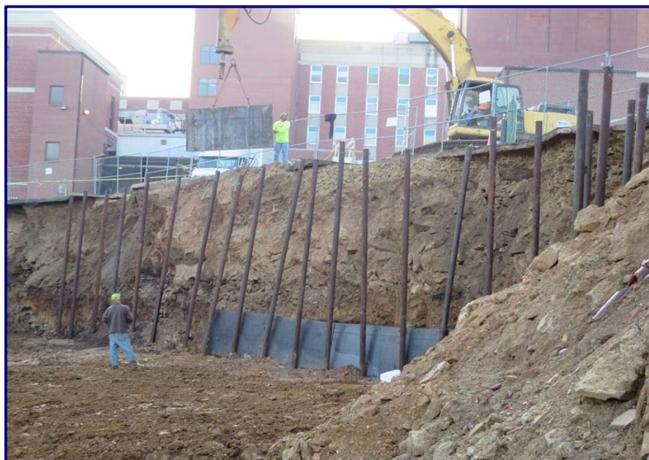
Figure 3. Lack of Personal Protective Equipment, Protection from Falling Debris, and Fall Arrest System
