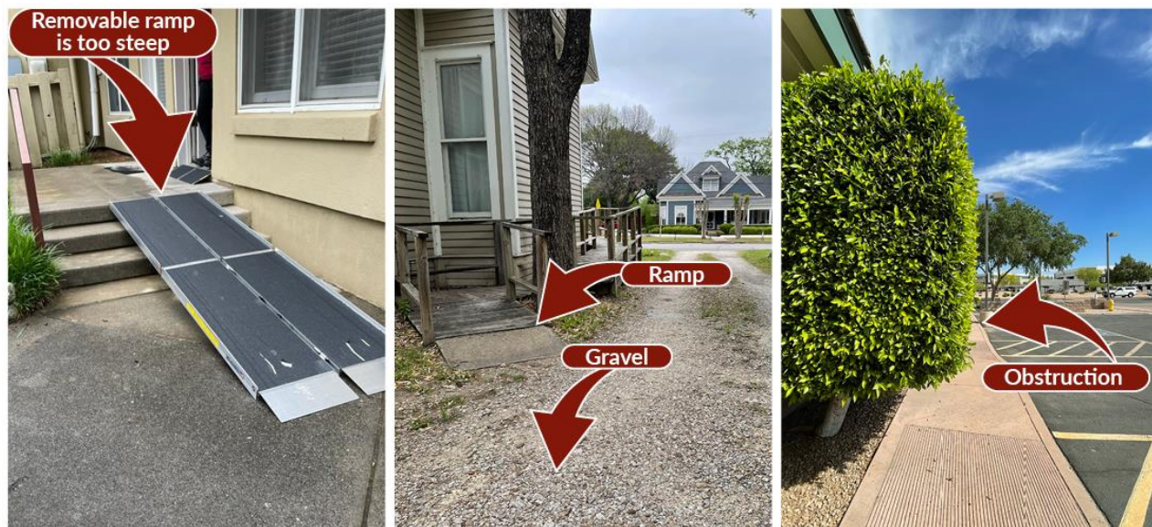
Figure 5. Accessibility deficiencies in contract exam facilities in Georgia (left), Texas (center), and Arizona (right).
