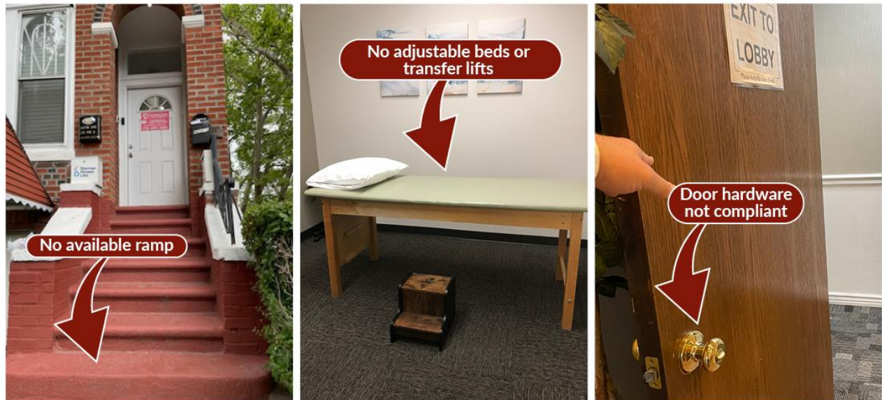
Figure 10. Noncompliant facilities in New York (left), Oregon (center), and Idaho (right).
