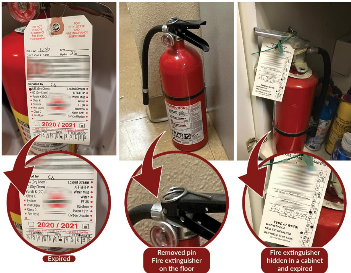
Figure 8. Fire extinguisher deficiencies in contract facilities in North Carolina (left), Arizona (center), and Texas (right).
