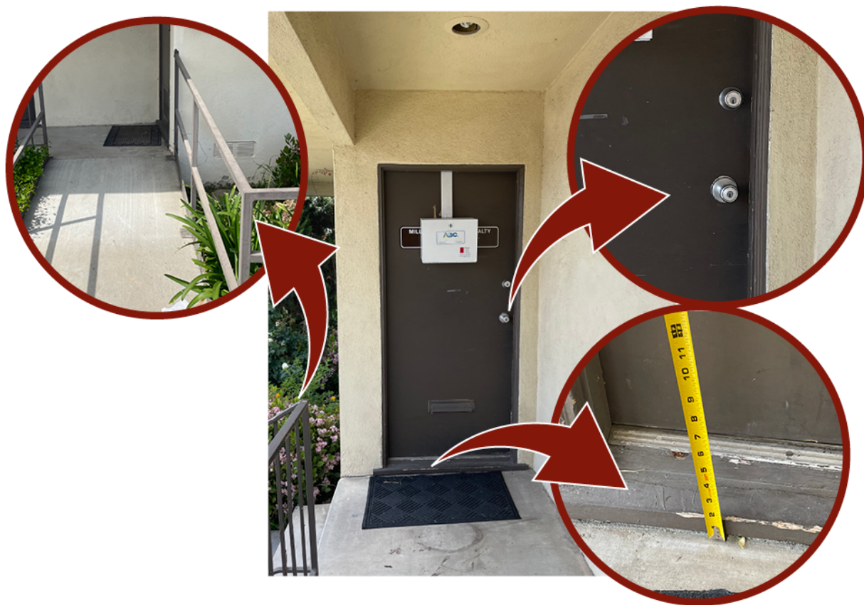
Figure 4. California contract exam facility with a handrail, door threshold, and door hardware that were not ADA compliant.
