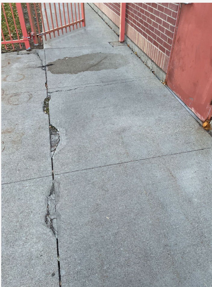
Figure 5. Damaged Concrete Near an Employee Entrance
