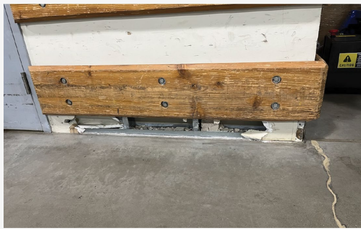
Figure 6. Missing Drywall on Workroom Floor
