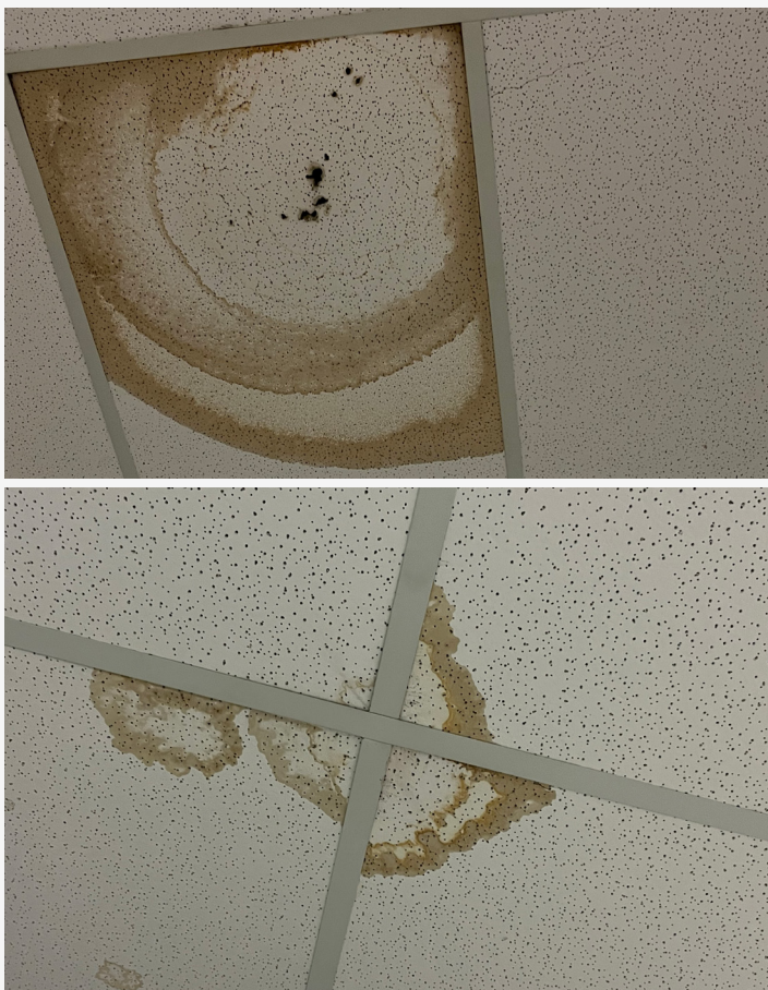
Figure 10: Stained Ceiling Tiles
