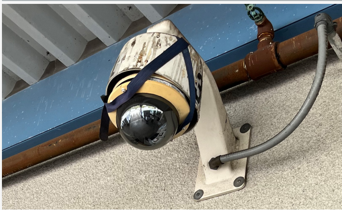
Figure 5: Broken Camera on Dock
