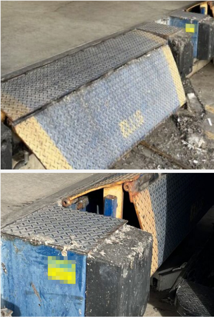
Figure 8. Broken Dock Lift
