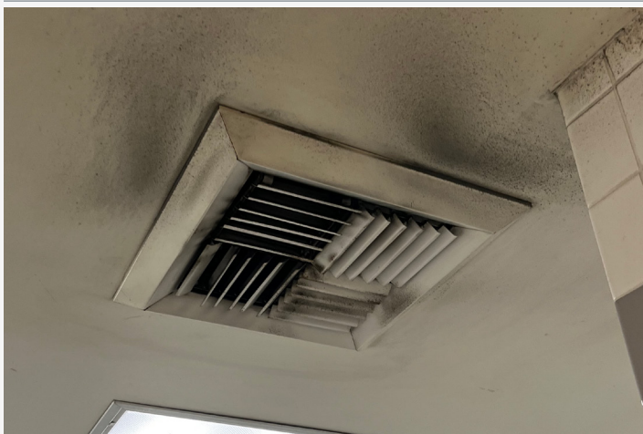
Figure 11: Dirty Air Vents
