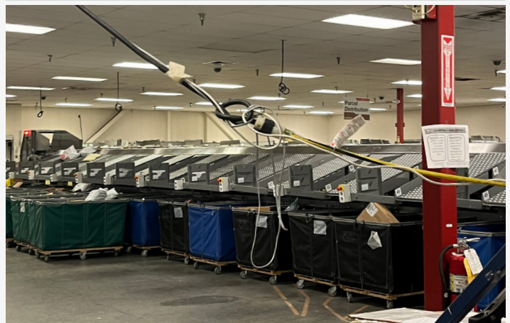
Figure 6. Electrical Cord Hanging Across Workroom Floor
