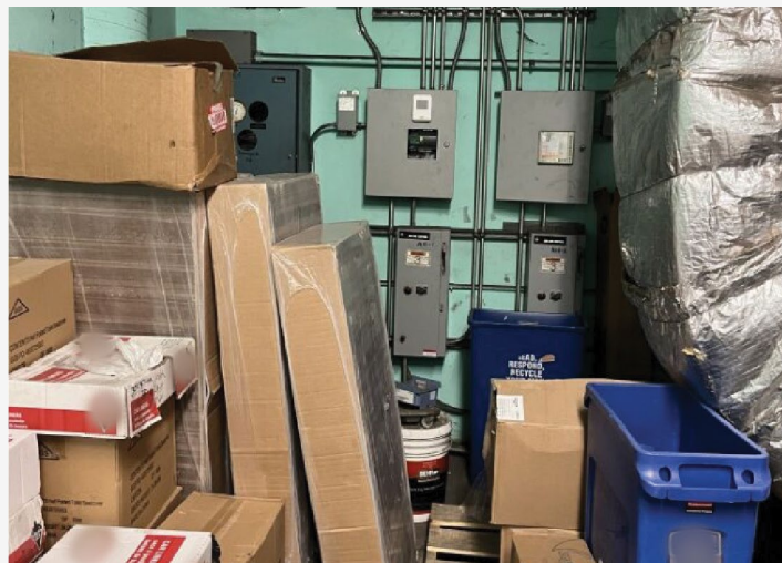
Figure 7. Blocked Electrical panels
