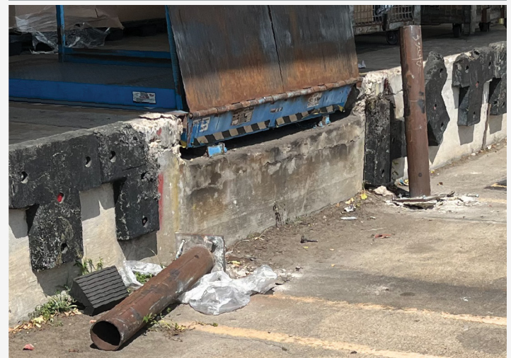
Figure 8. Broken Safety Poles at Loading Dock
