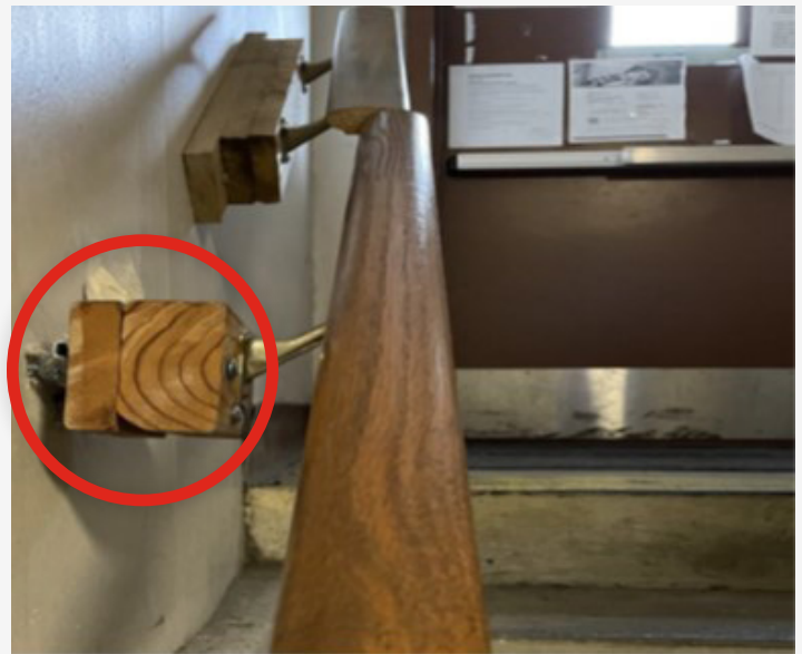
Figure 5. Loose Handrail on Staircase
