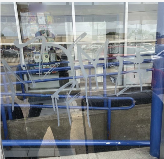
Figure 11. Graffiti on the Building's Front Retail Side
