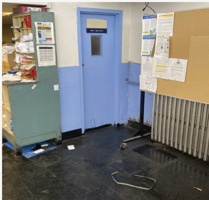
Figure 7. Unblocked Postal Inspection Service Door
