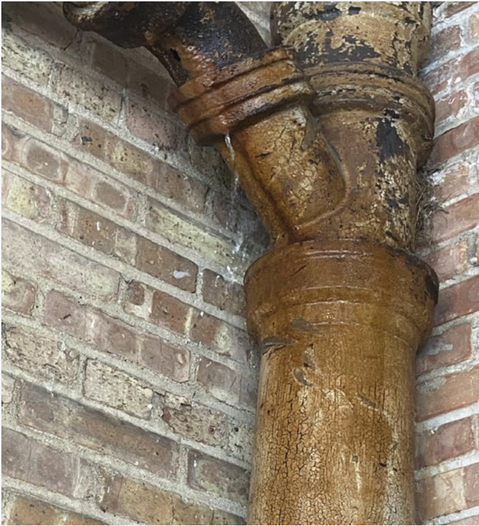
Figure 10. Leaking Pipe on the Loading Dock
