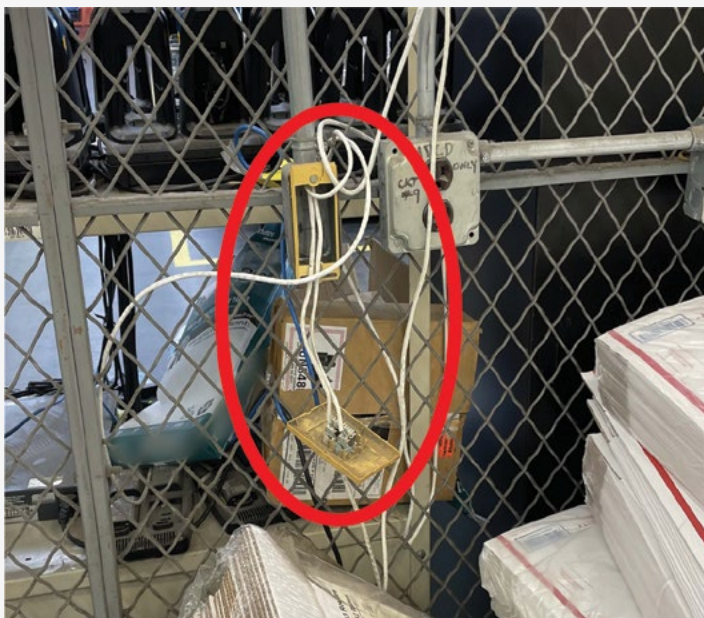
Figure 5. Exposed Wiring in the Registry Cage
