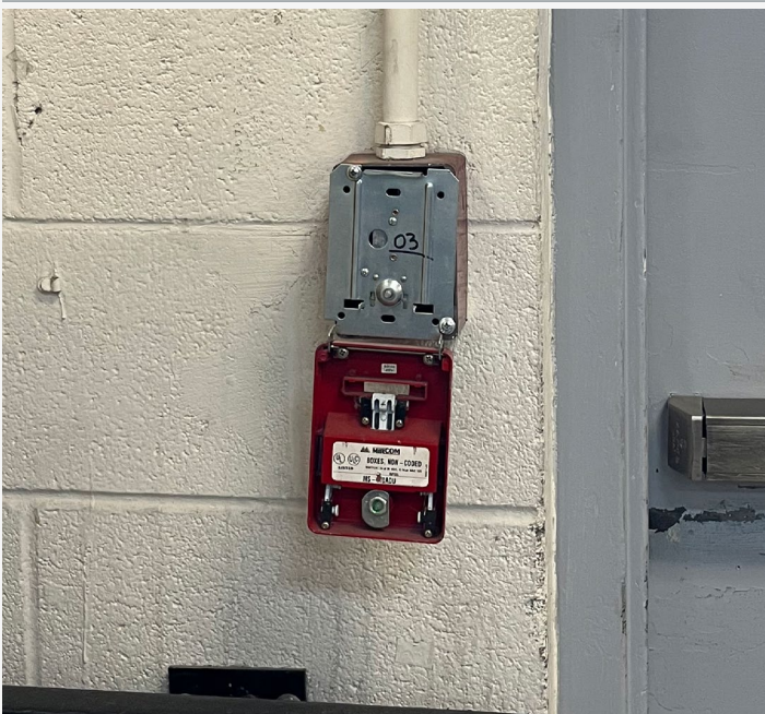
Figure 2. Broken Manual Fire Alarm Pull
