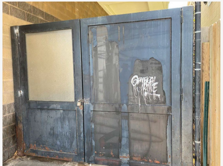
Figure 5. Graffiti on the Front, Retail Side
