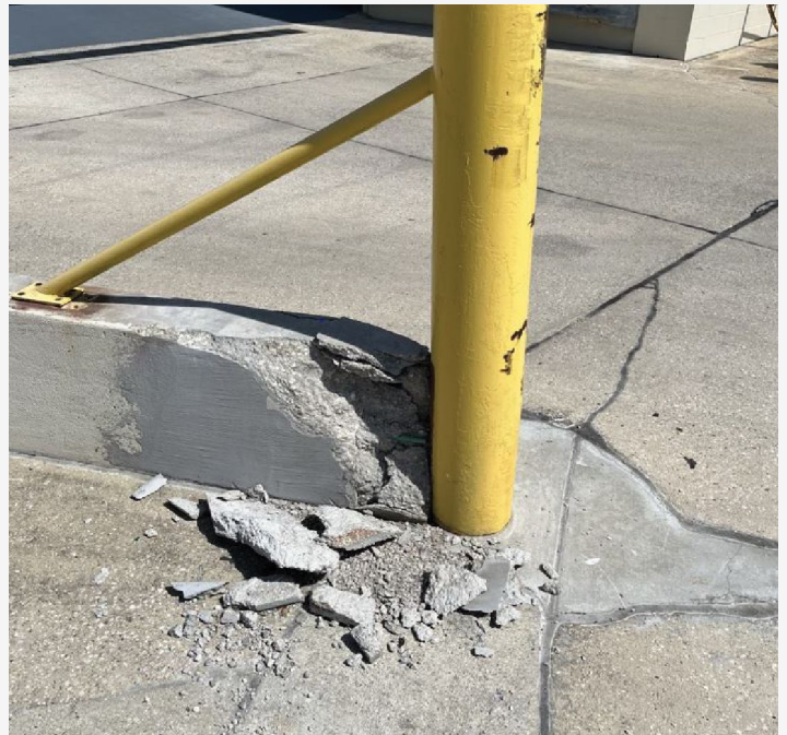
Figure 4. Crumbling Concrete Base Near Dock
