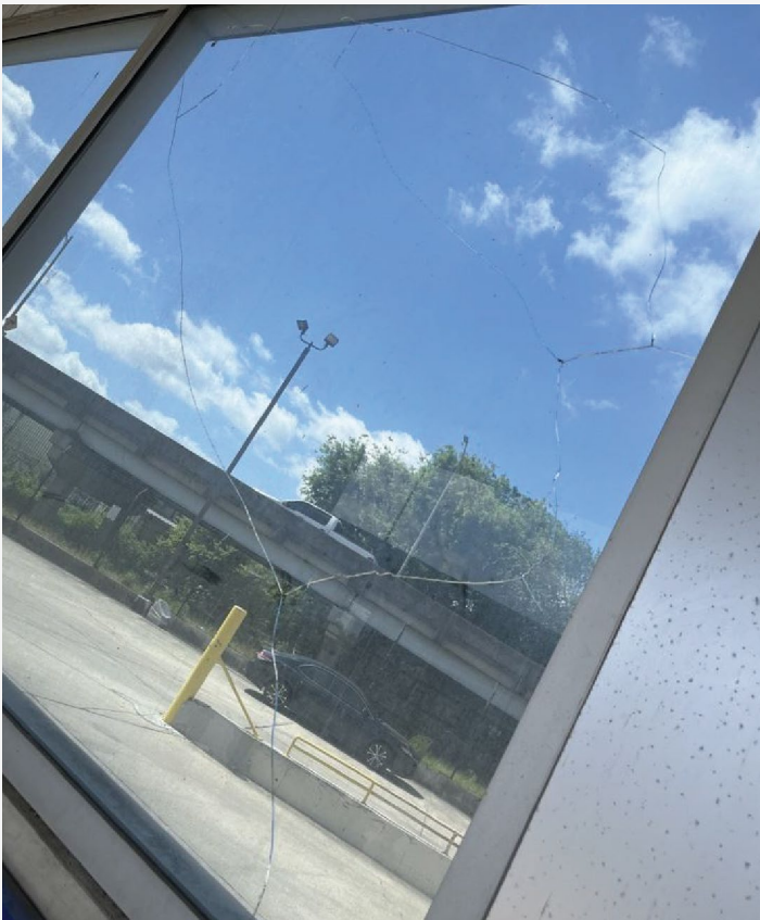
Figure 3. Cracked Window on Workroom Floor
