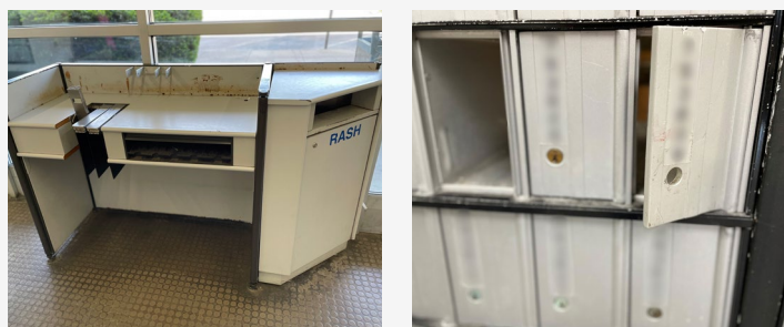
Figure 5. Damaged Counter and PO Boxes in the Customer Retail Area
