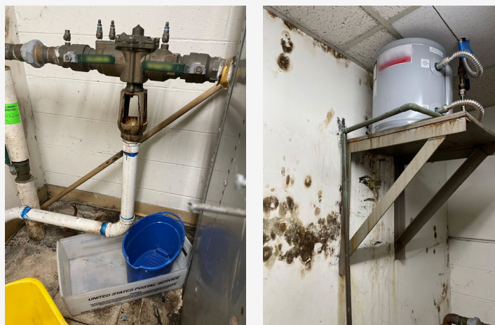
Figure 4. Leaky Pipes and Potential Mold in Maintenance Room
