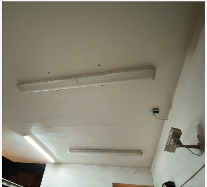
Figure 4. Non-working Dock Lights
