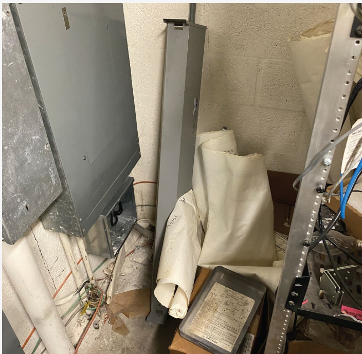
Figure 3. Blocked Electrical Panel
