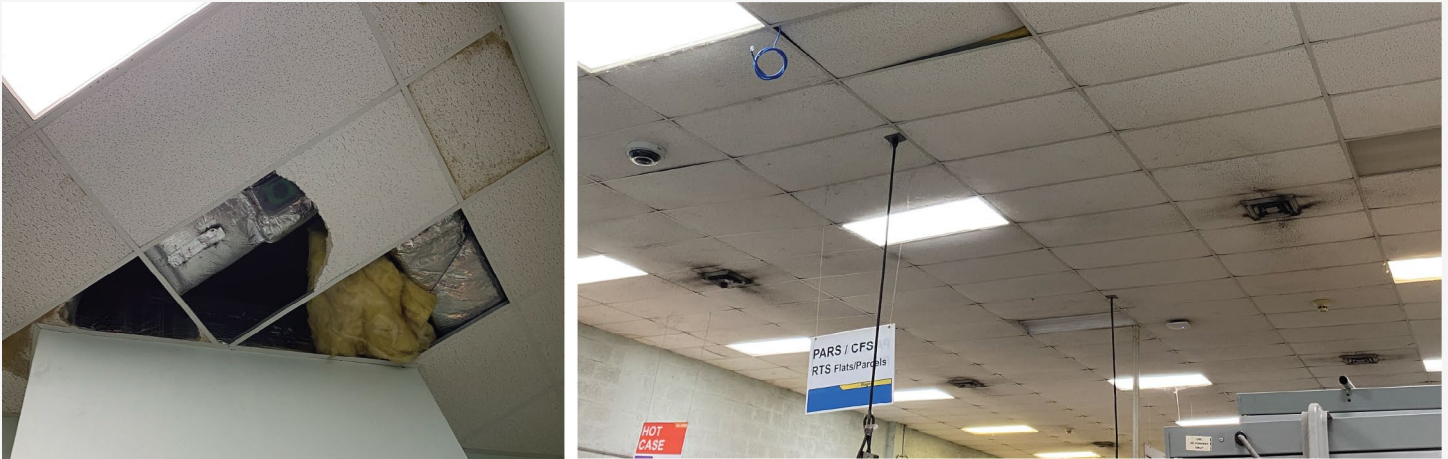
Figure 5. Damaged, Missing, and Stained Ceiling Tiles and Dirty Air Vents
