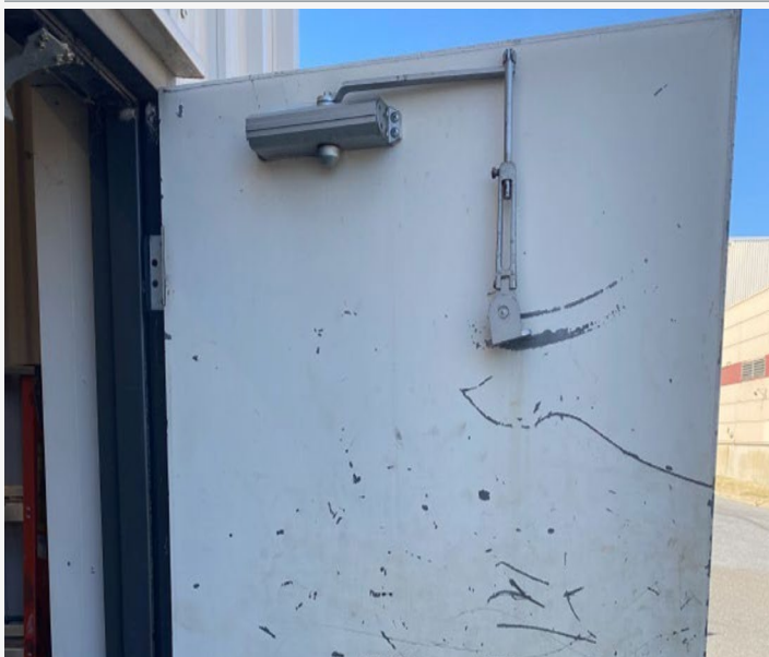
Figure 8. Broken Door Closure
