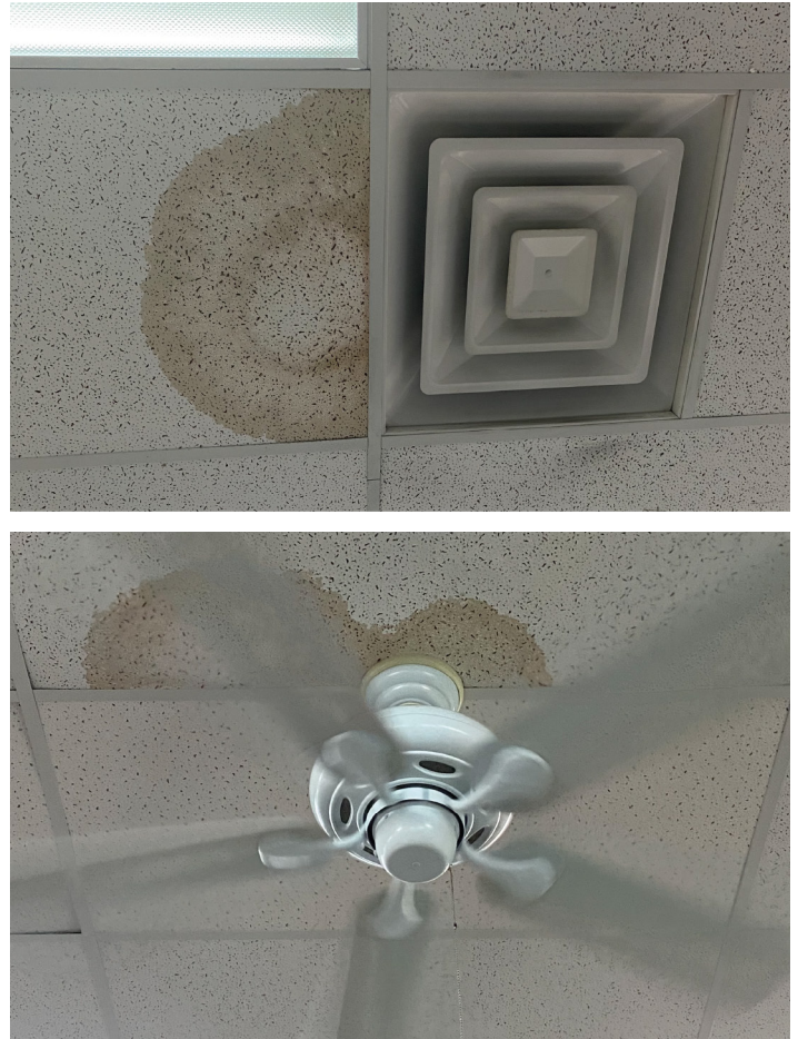
Figure 3. Stained Ceiling Tiles at McDonough MPO
