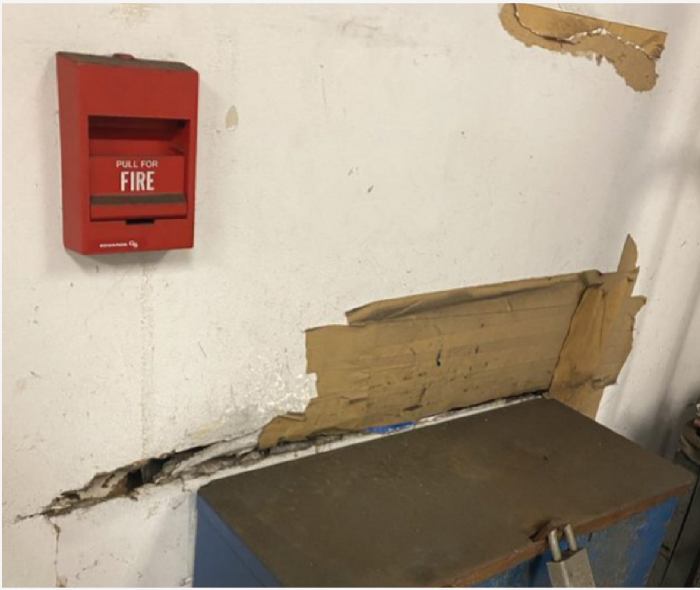
Figure 5. Damaged Wall Near Dock Area
