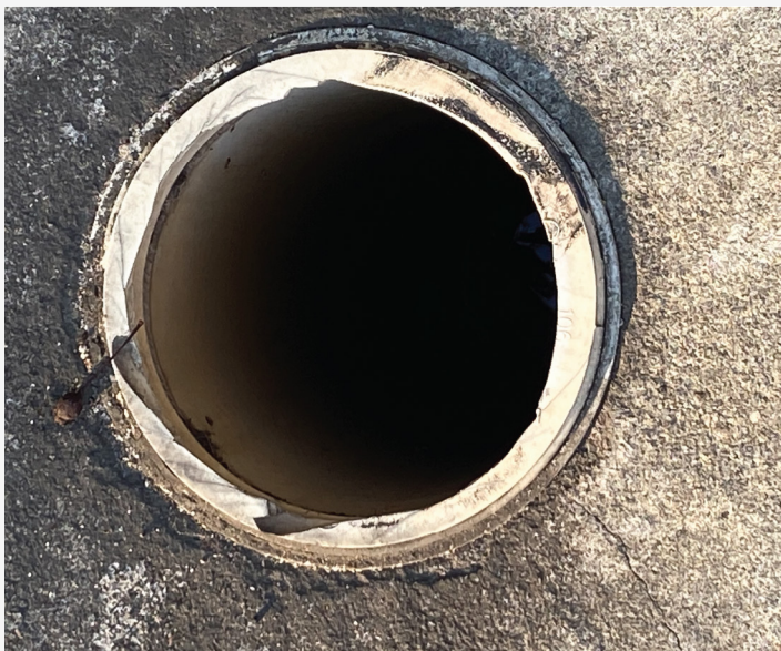
Figure 2. Uncovered Drainage Hole in Postal Vehicle Lot
