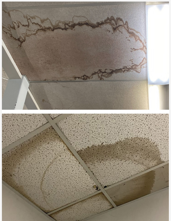
Figure 4. Examples of Stained Ceiling Tiles
