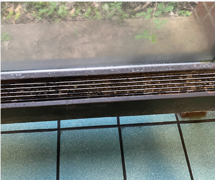
Figure 6. Dirty Heat Vent in Customer Lobby
