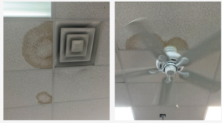
Figure 5. Stained Ceiling Tiles
