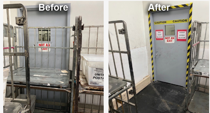
Figure 4. Blocked Inspection Service Door
