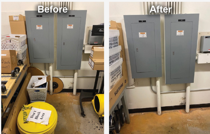
Figure 3. Blocked Electrical Panels
