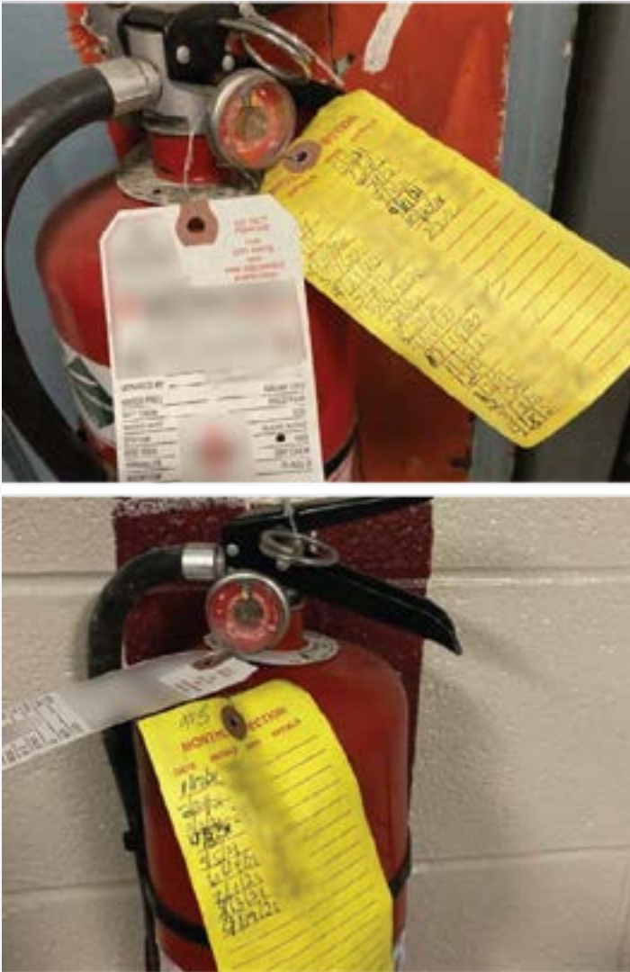
Figure 2. Missing Annual and Monthly Fire Extinguisher Inspections
