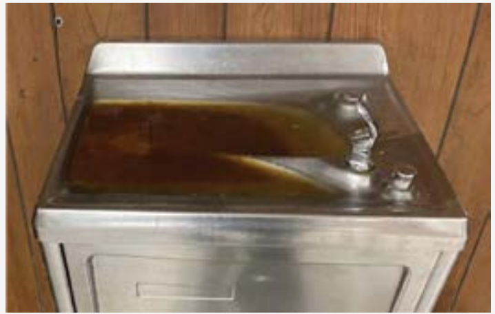
Figure 3. Broken Water Fountain
