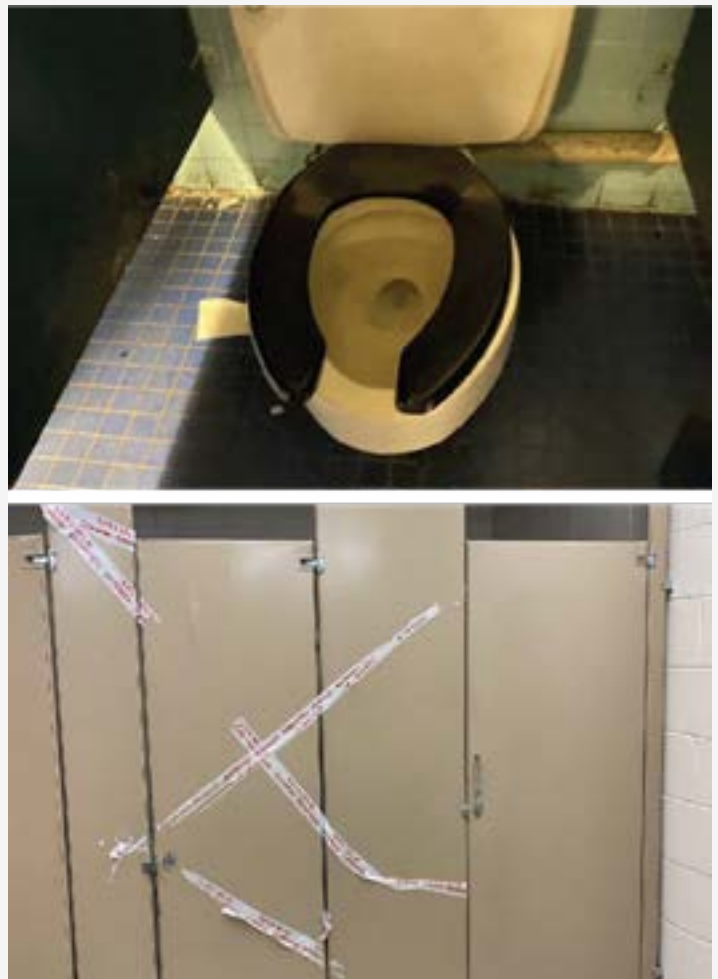
Figure 4. Inoperable Toilets in the Men's and Women's Restrooms
