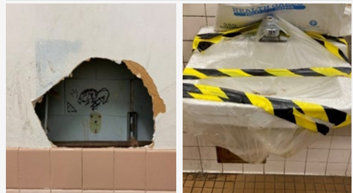
Figure 3. Damaged Wall in Men's Bathroom and Inoperable Fixture in Women's Bathroom
