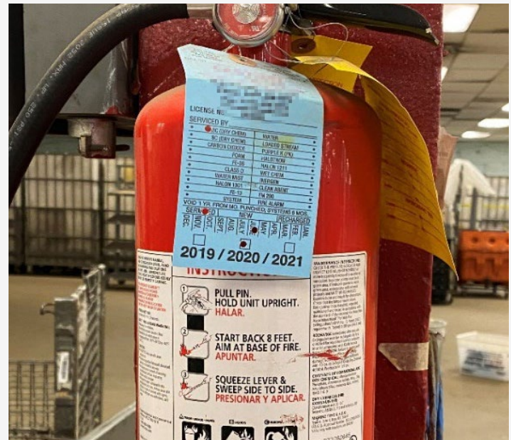
Figure 2. Fire Extinguisher Missing Annual Inspection
