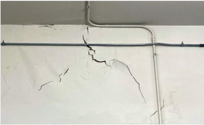
Figure 10. Cracks in Work Room Walls
