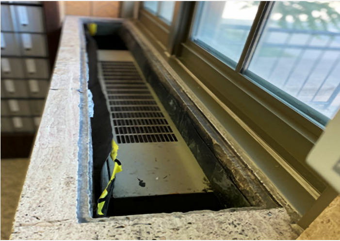
Figure 11. Missing Heating Vent Cover
