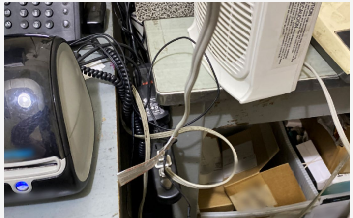
Figure 7. Appliances Plugged Into a Power Strip
