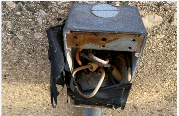
Figure 8. Electrical Box with Exposed Wires
