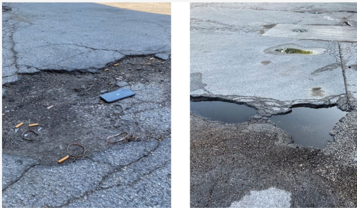
Figure 15. Potholes near the Loading Dock
