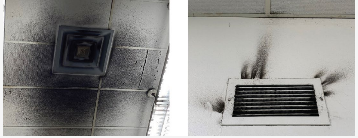
Figure 12. Dirty Air Vents and Ceiling Tiles
