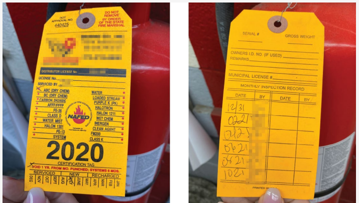
Figure 13. Missing Annual and Monthly Fire Extinguisher Inspections
