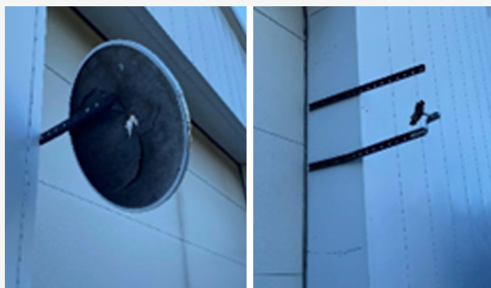
Figure 5. Broken or Missing Safety Mirrors
