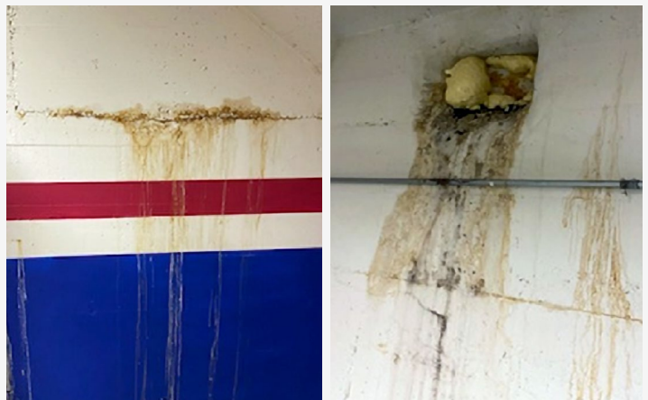
Figure 9. Water-Stained Walls in the Basement
