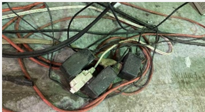
Figure 4. Excessive Electrical Plugs
