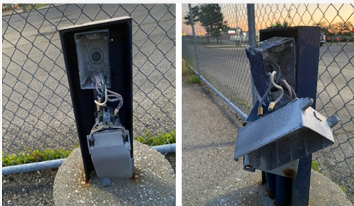
Figure 3. Damaged Exterior Outlets
