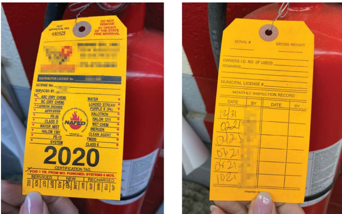
Figure 3. Missing Annual and Monthly Fire Extinguisher Inspections
