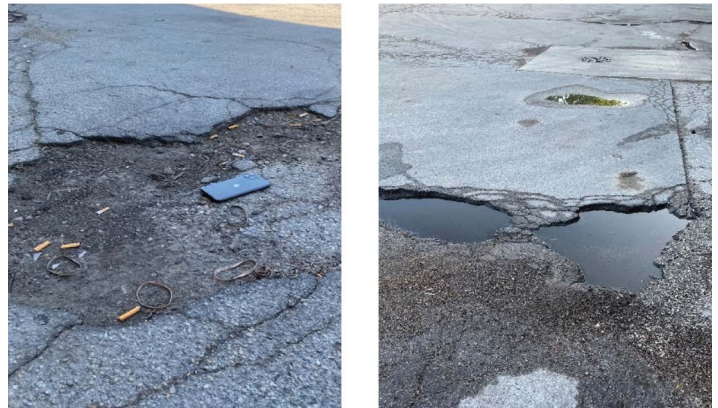
Figure 5. Potholes near the Loading Dock
