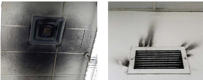
Figure 2. Dirty Air Vents and Ceiling Tiles
