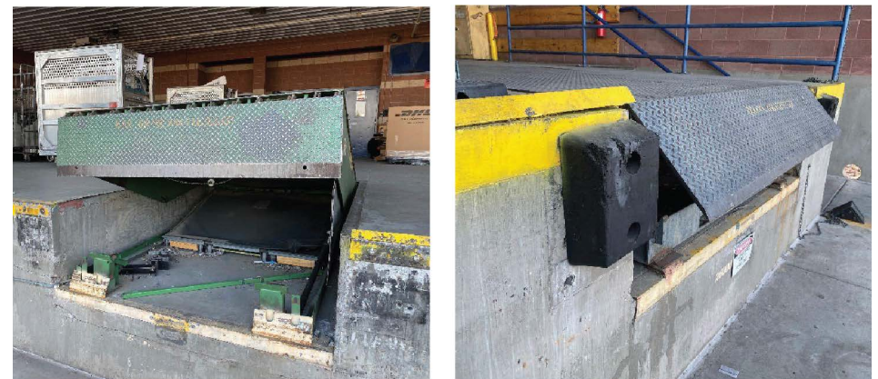
Figure 4. Broken Dock Lifts
