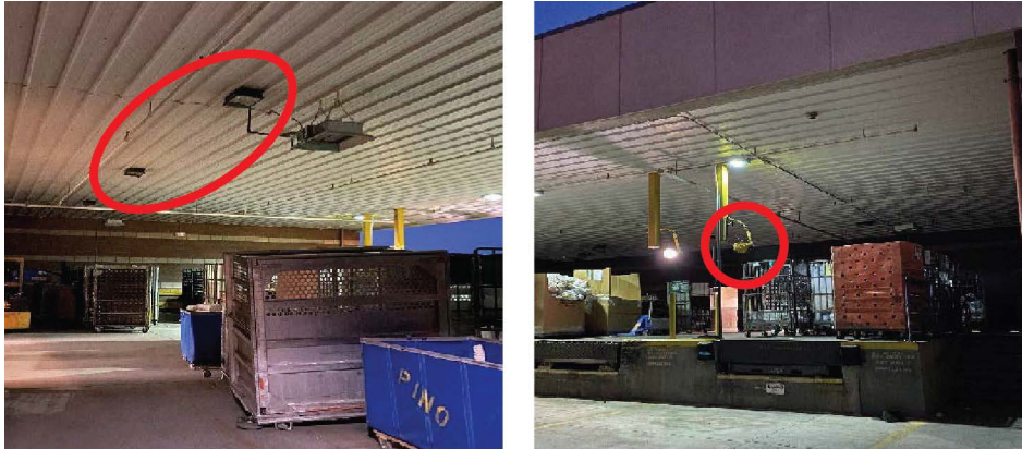
Figure 5. Non-Working Dock Lights
