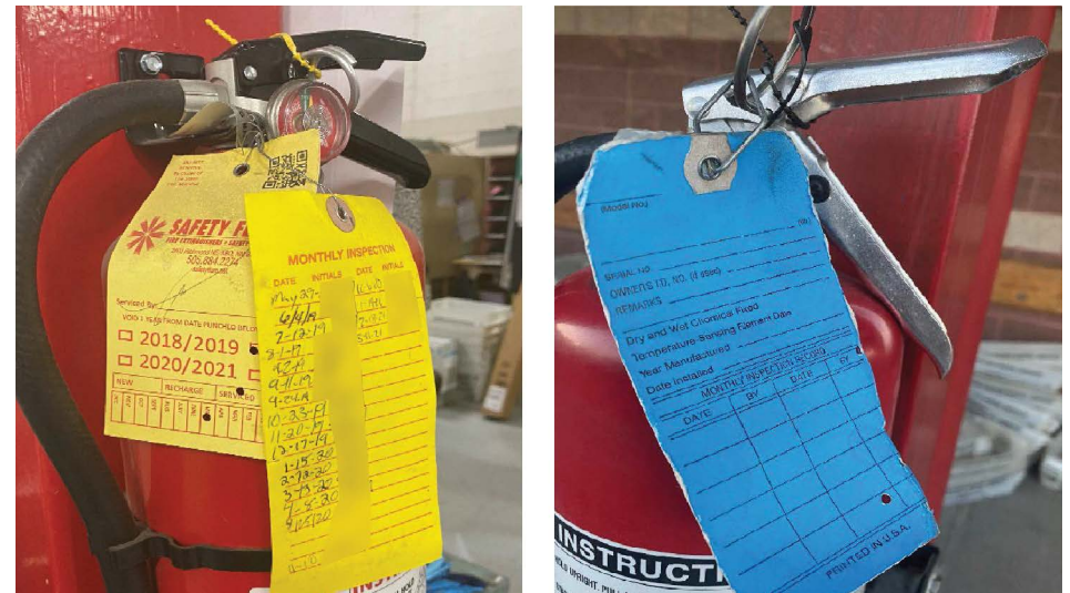
Figure 3. Fire Extinguishers Missing Annual or Monthly Inspections
