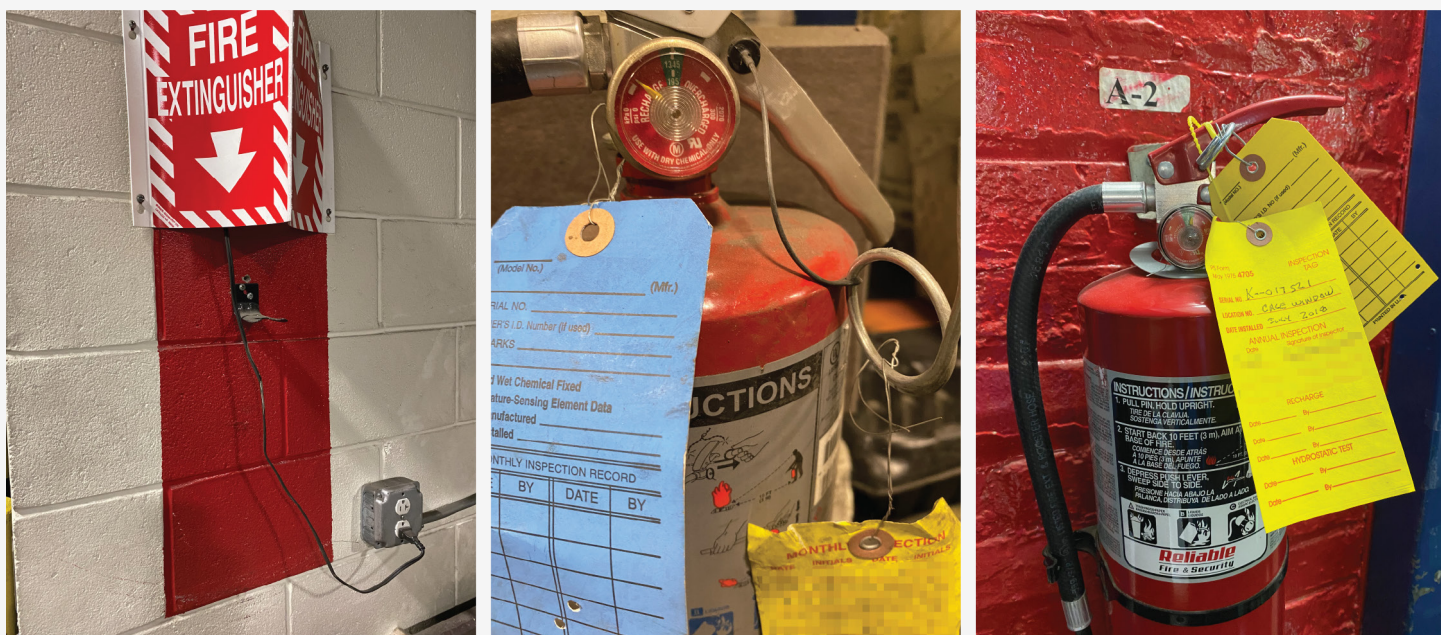
Figure 6. Missing and Underserviced Fire Extinguishers
