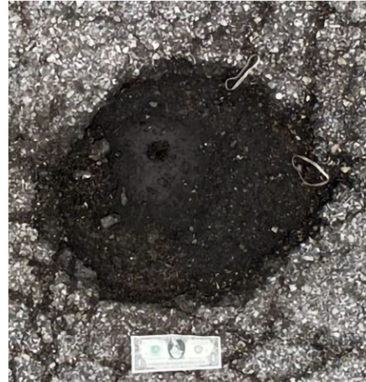
Figure 23. Pothole in Employee Parking Lot
