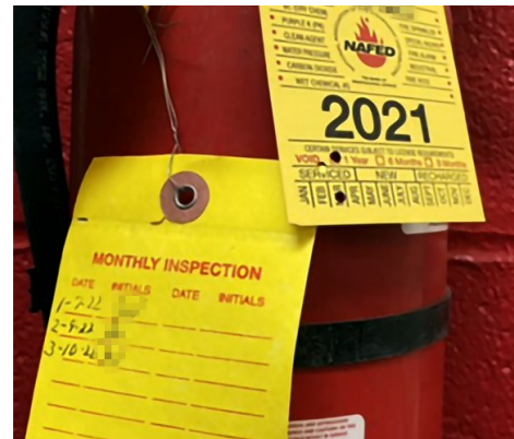
Figure 20. Example of Fire Extinguisher Missing Inspections
