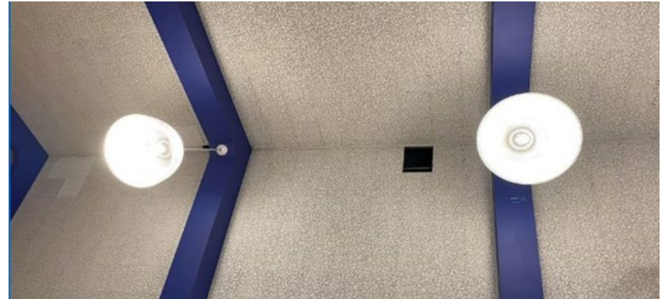
Figure 3. Missing Ceiling Tile
