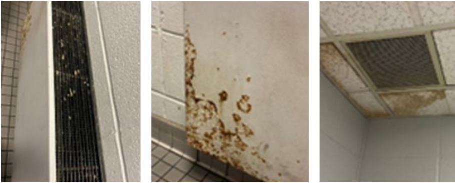
Figure 5. Dirty/Rusted Air Vent and Stained Tile in Men's Restroom
