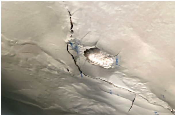
Figure 18. Walls With Water Damage
