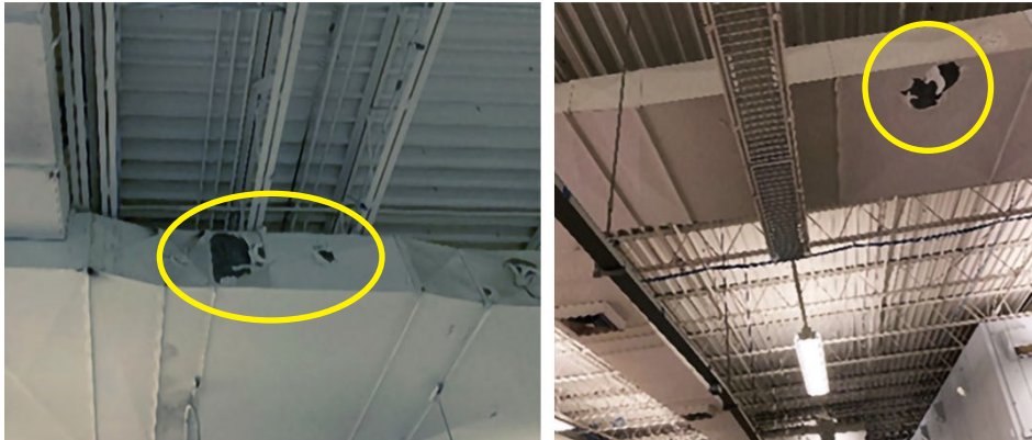
Figure 9. Peeling Paint Above Workroom Floor
