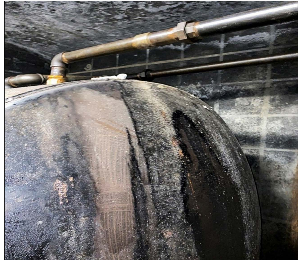
Figure 3. Example of Leaking AST
