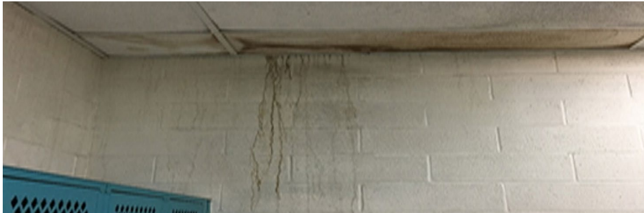
Figure 1. Damaged Ceiling Tiles Near the Manager’s Office and Women’s Restroom
