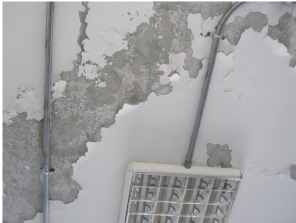
Photo 2 - Paint Peeling off Classroom Ceiling
