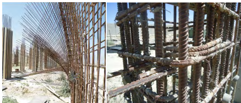
Tilted columns, sagging reinforcing rods, and faulty rebar at the JCIP courthouse construction site in Parwan province, Afghanistan.
