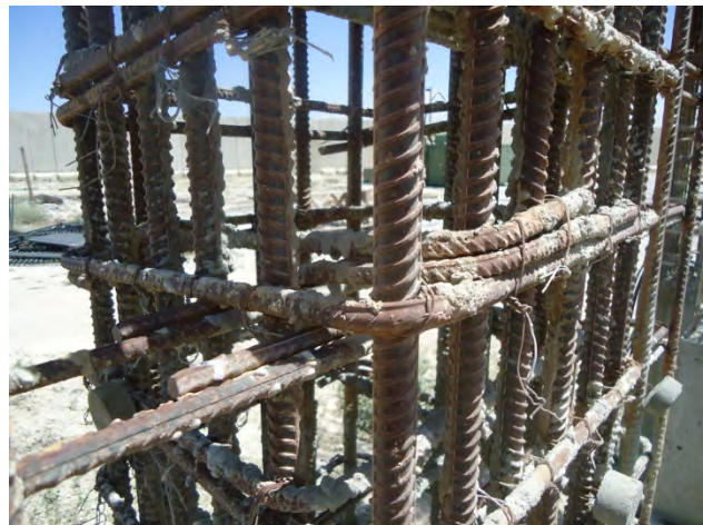
Photo 3 - Rebar Is Tied Together Instead of Welded
