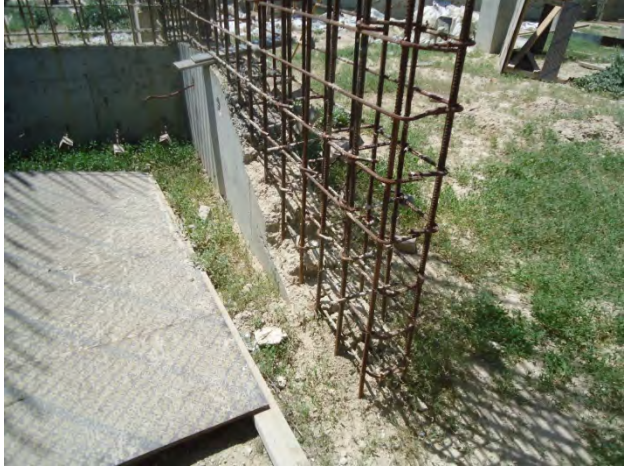
Photo 2 - Incomplete Concrete Pour of Wall Could Result in Structural Failure
