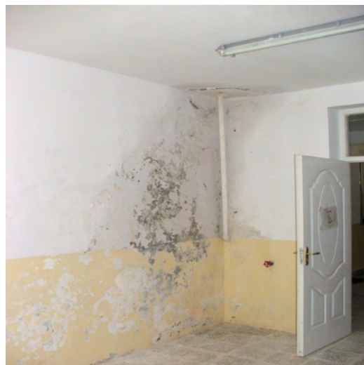
Photo 2 - Leaky Roof Damages Ceilings and Walls
