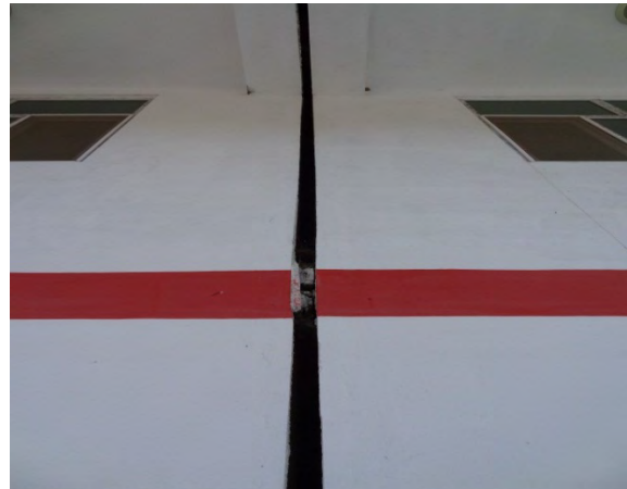
Photo 3 - Excessively Wide Expansion Joint
