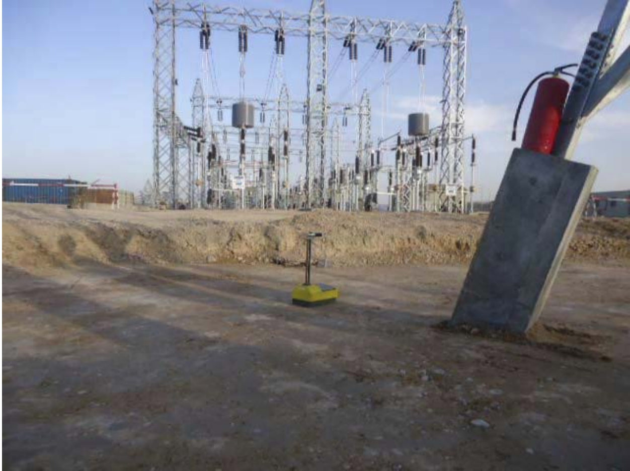
The photograph above is of the Durai Substation, which was rebuilt under the scope of CLIN 2. The photograph was taken by Horwath MAK, Crowe Horwath LLP's Afghanistan affiliate, during in-country observation and inspection activities pertaining to the audit of BVSPC's Special Purpose Financial Statement.
