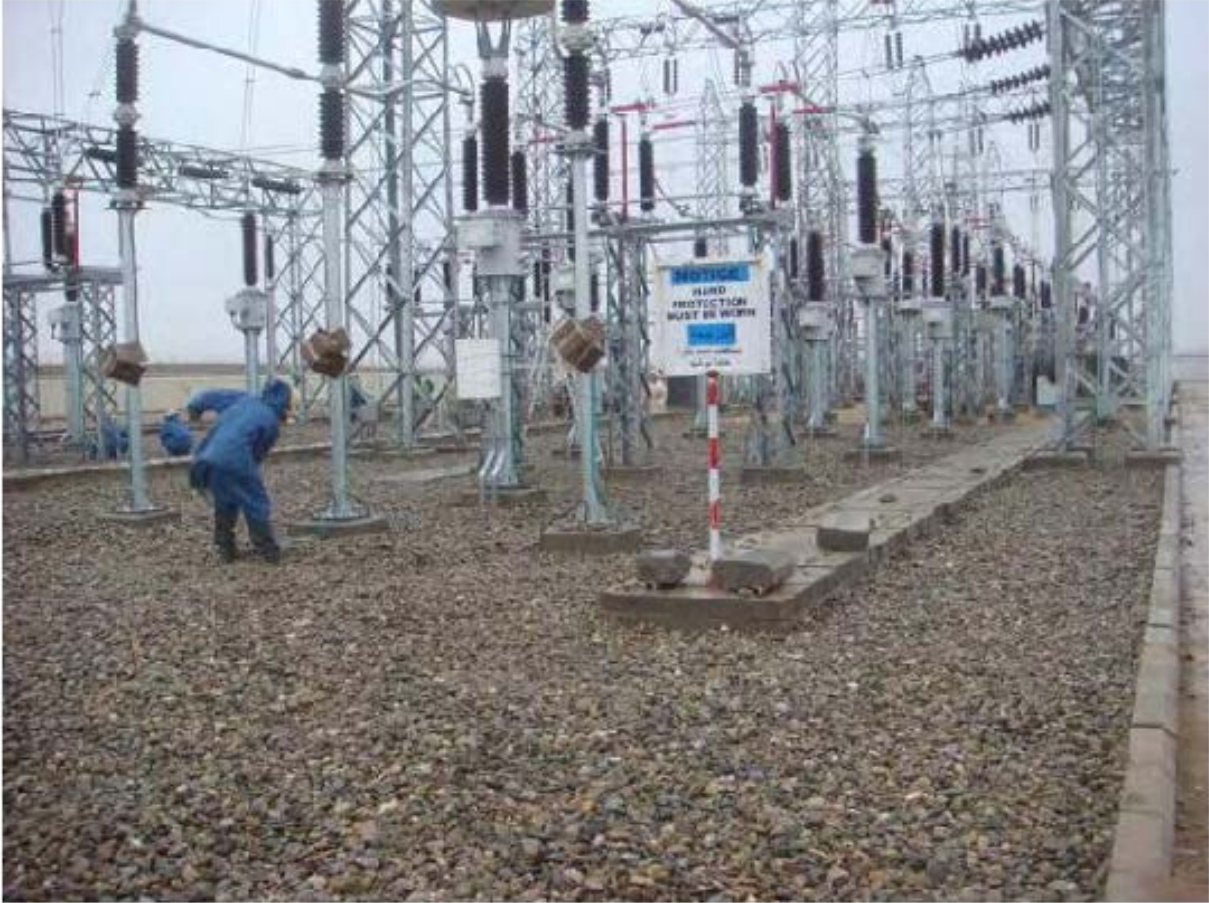
The photograph above is of the Durai Substation, which was rebuilt under the scope of CLIN 2. The photograph was taken by Horwath MAK, Crowe Horwath LLP's Afghanistan affiliate, during in-country observation and inspection activities pertaining to the audit of BVSPC's Special Purpose Financial Statement.
