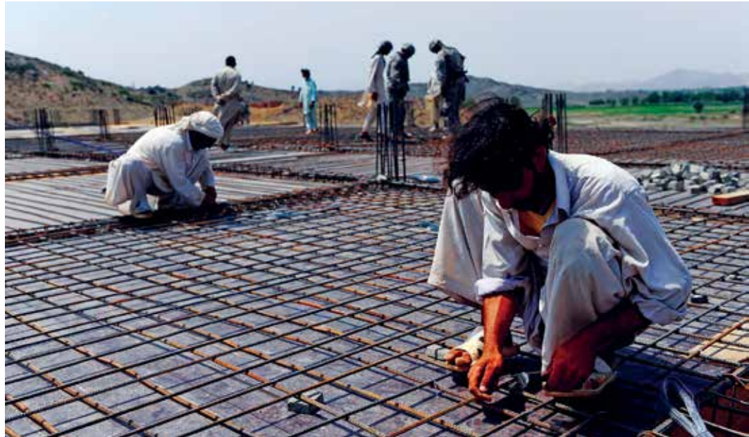
Members of Khost PRT check the quality of the work done on the Hassan Khot school roof on July 3, 2010. (U.S. Air Force photo by Senior Airman Julianne M. Showalter)
