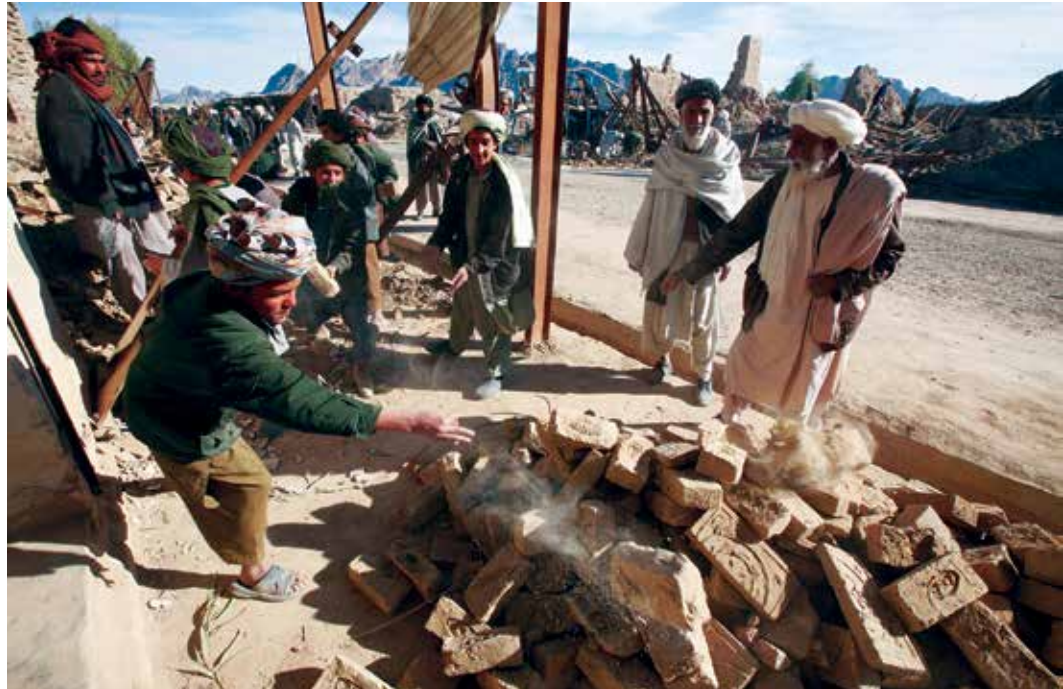
Using CERP funds, Afghan men rebuild markets in Now Zad District, Helmand Province, on December 17, 2009. (U.S. Marine Corps photo by Cpl. Daniel M. Moman)
