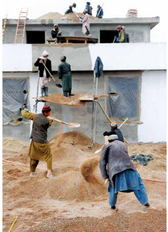
Afghan laborers move dirt and gravel up a series of platforms to the roof of a new prison in Tarin Kowt, Uruzgan Province, on February 1, 2011. (U.S. Air Force photo by 1st Lt. Matt Schroff)
