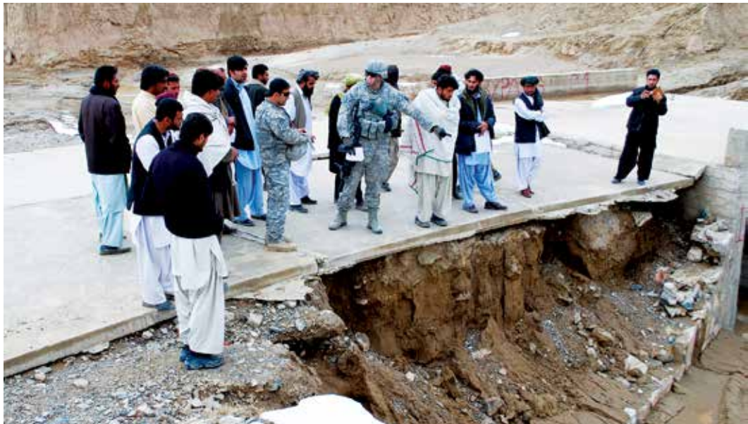
U.S. Air Force Tech. Sgt. Latha Caillouette, a PRT Zabul engineer, shows contractors erosion control repairs that are needed at a bridge in Shah Joy District, Zabul Province, on March 4, 2011. (U.S. Air Force photo by 1st Lt. Brian Wagner)
