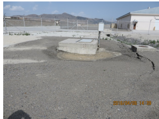
Photo 2 - Ground Settlement and Water Pooling Around the Lift Station
