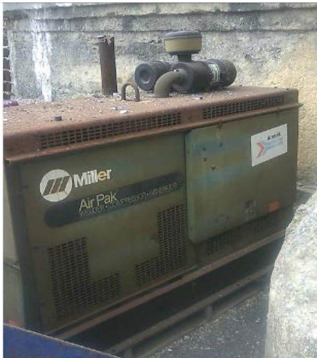
Figure 2. A Generator the Department Has Not Inspected Since 2015
