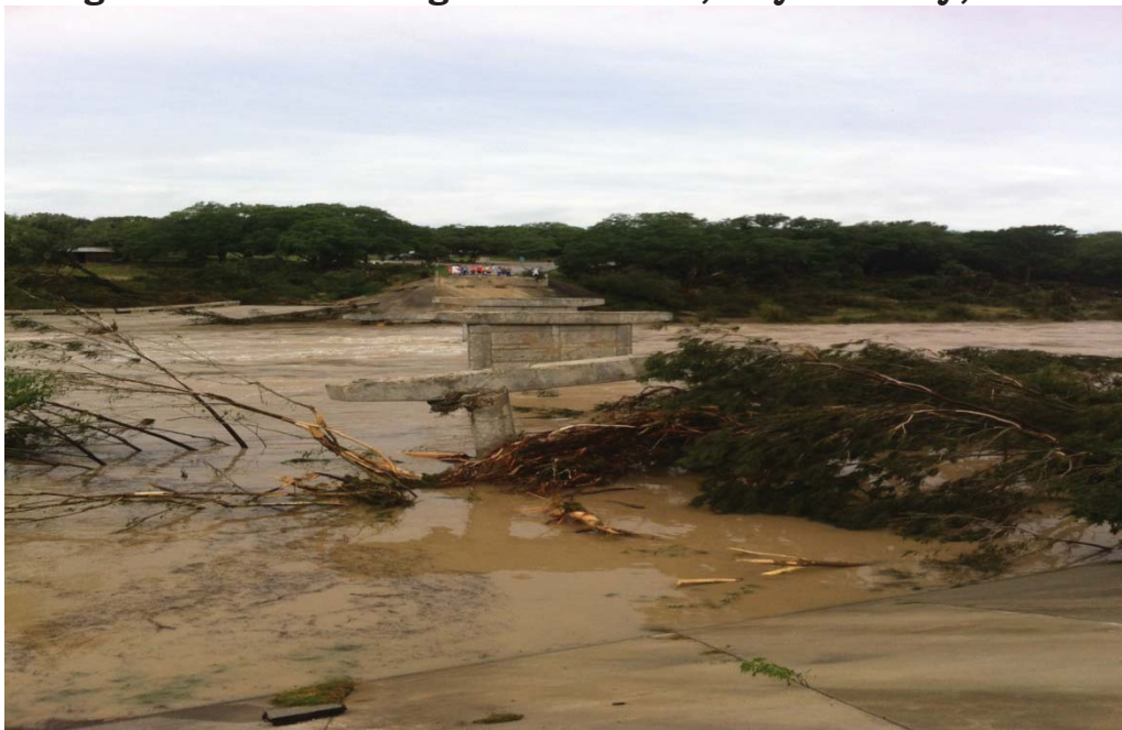
Figure 1: Fisher Bridge Washed Out, Hays County, Texas
