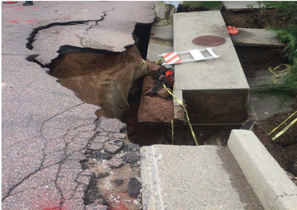
Figure 1: Culverts Washed Out in Colorado Springs, CO
