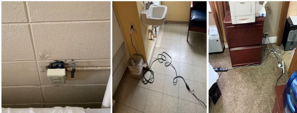
Photograph 11 (left): Electrical outlet pulled off the wall exposing electrical wires.
