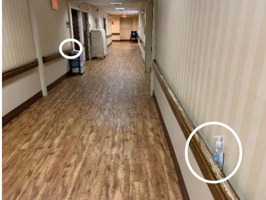
Photograph 8 (left): Unsecured hand rub dispensers.
