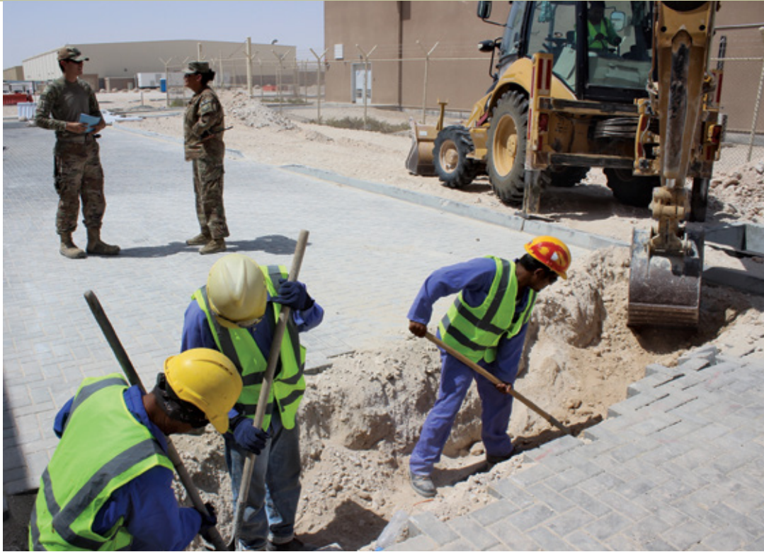
Construction workers dig a trench at Al Udeid Air Base, Qatar. (DoD photo)
