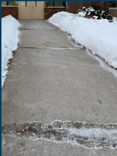
Deterioration of an External Walkway
