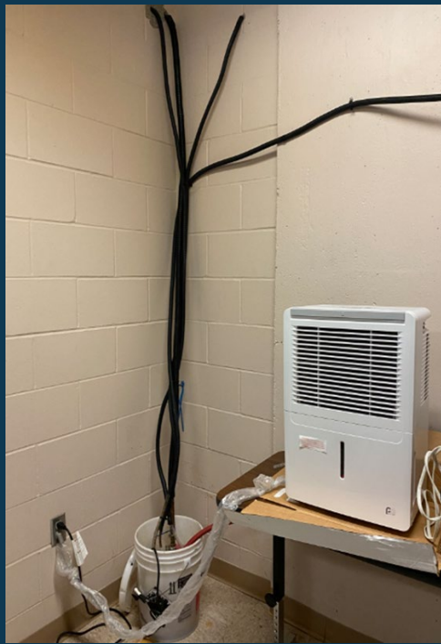
Makeshift Sump Pump in Evidence Room
