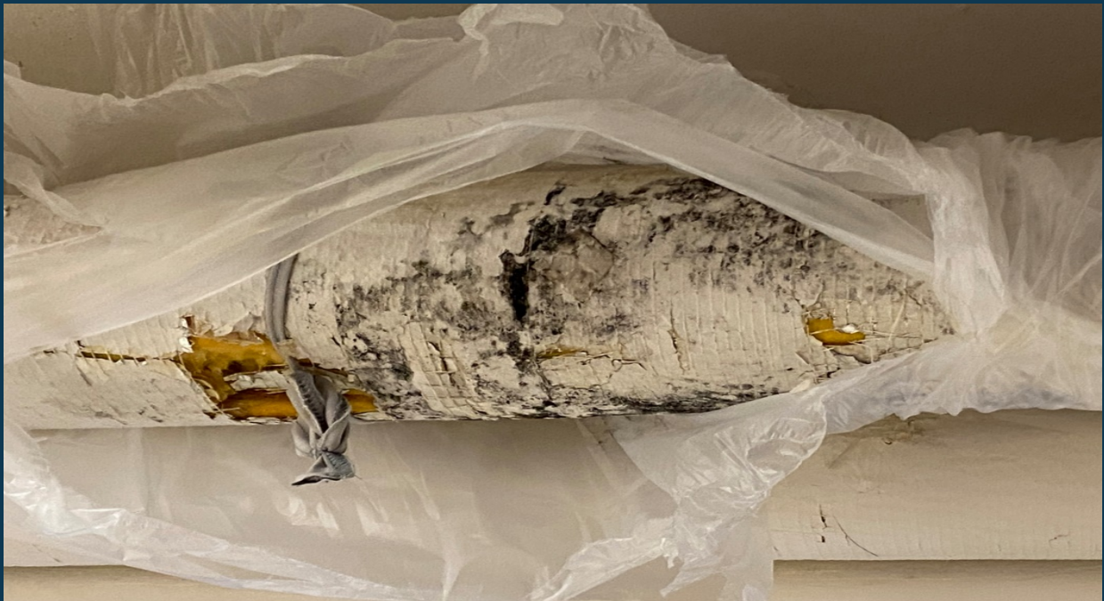
Pipe Uncovered in a Basement Housing Floor. To better assess the pipe's condition, the OIG cut open the plastic sheeting that had been covering the pipe.
