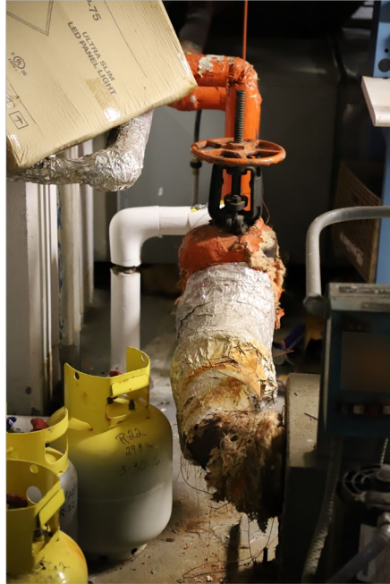
Old insulation covering water and steam pipes (brand name blurred in photo)
