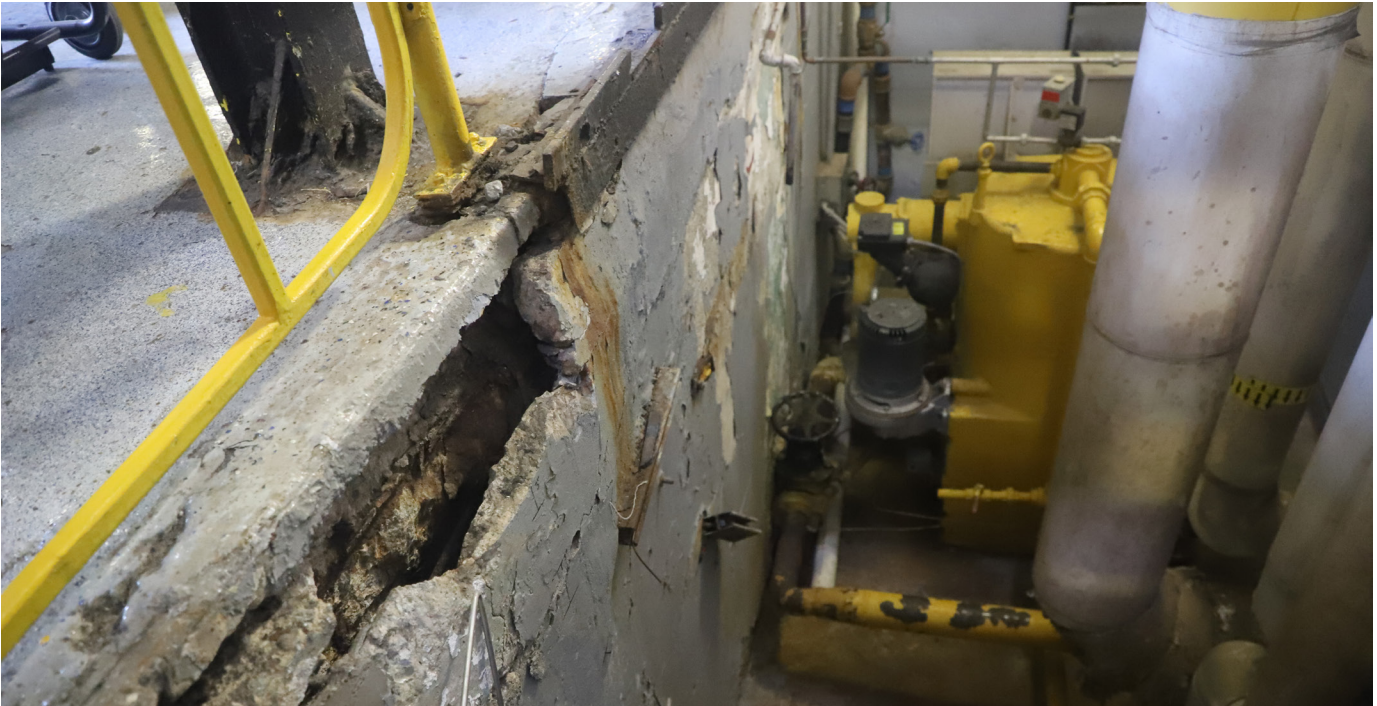
Cracking and separation in the powerhouse floor, where the boilers are located, FCI Terminal Island. Source: OIG, April 2022
