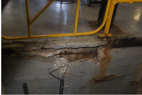
Deterioration in the pit wall
