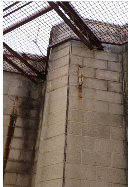
Damaged wall in the rooftop recreation area
