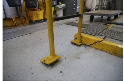
Cracking and separation (brand name blurred in photo)
