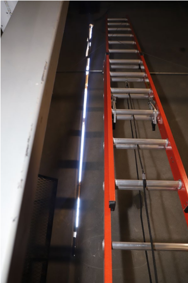
Crack in exterior wall with daylight visible
