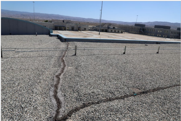
The library has extensive damage, including the roof
