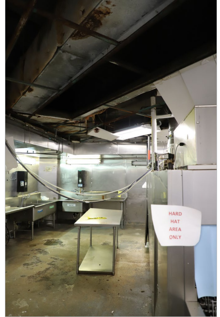
Food Services in complete disrepair
