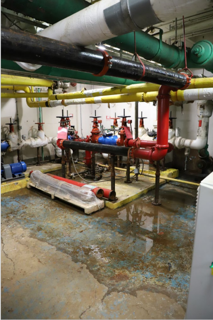
Flooded pump room
