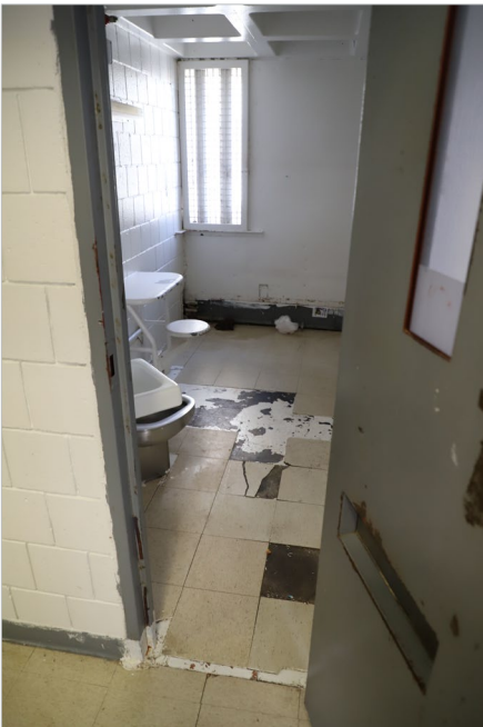
Cell in need of repairs
