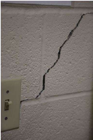
Crack near a light fixture
