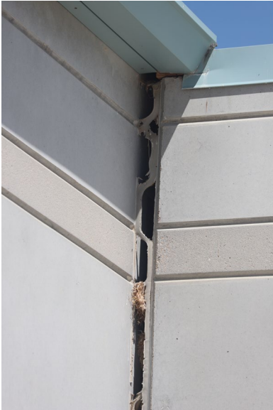
Significant separation between adjoining walls
