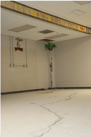
Crack in the library floor
