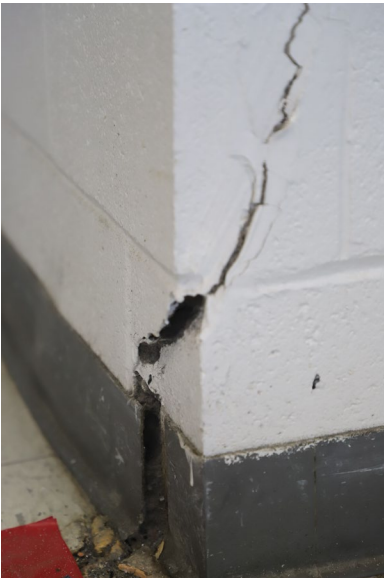
Crack from the floor to the wall
