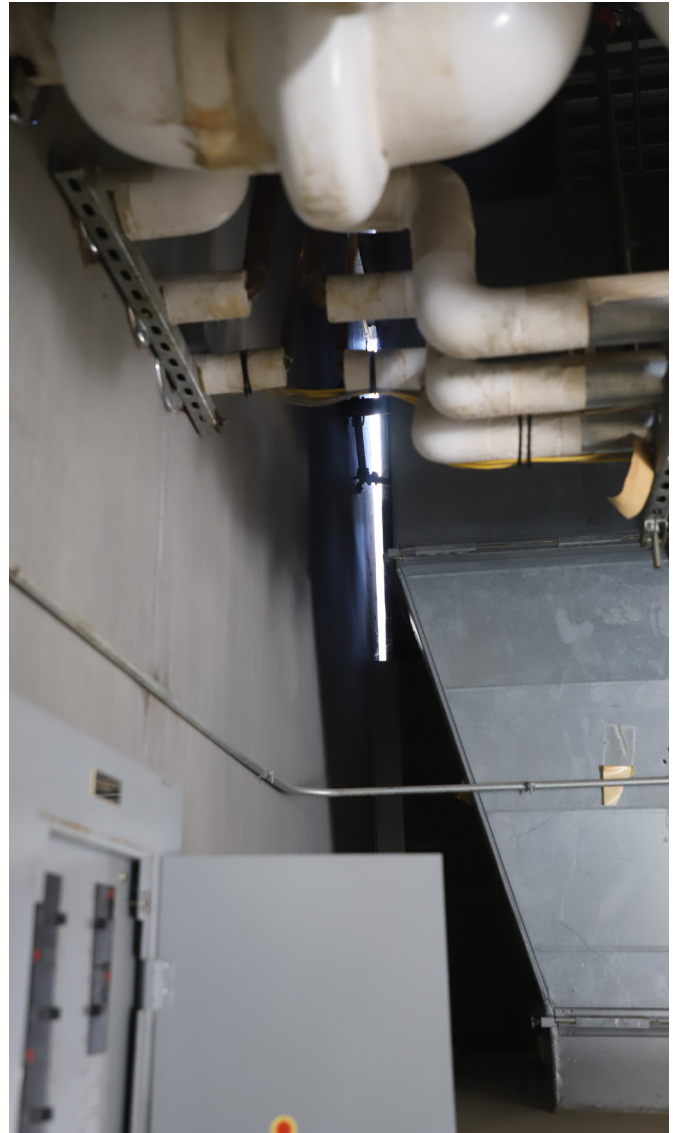
Wall separation in the mechanical room allows daylight to be seen from the building's interior, CI Taft. Source: OIG, April 2022 (institution closed at time of photo)
