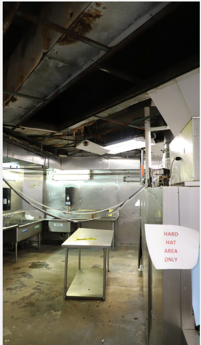
The Food Services area in complete disrepair, including exposed and corroded rebar in the ceiling, MCC New York. Source: OIG, March 2022 (institution closed at time of photo)
