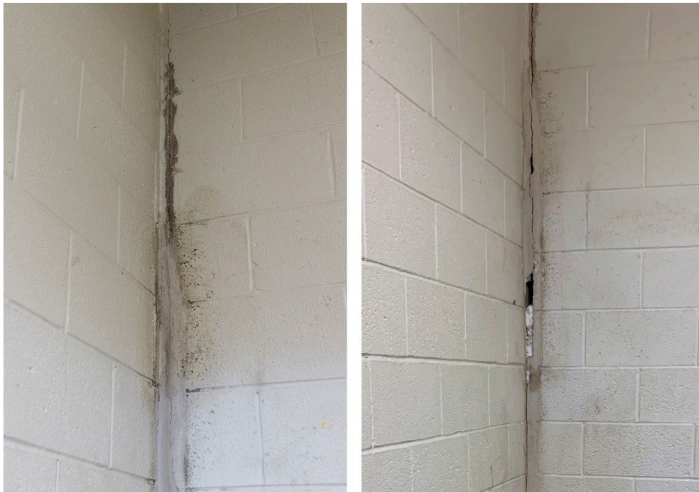
Figure 1: Crack in the Wall Between Adult and Juvenile Holding Cells, Observed in 2015 (Left) and 2022 (Right)
