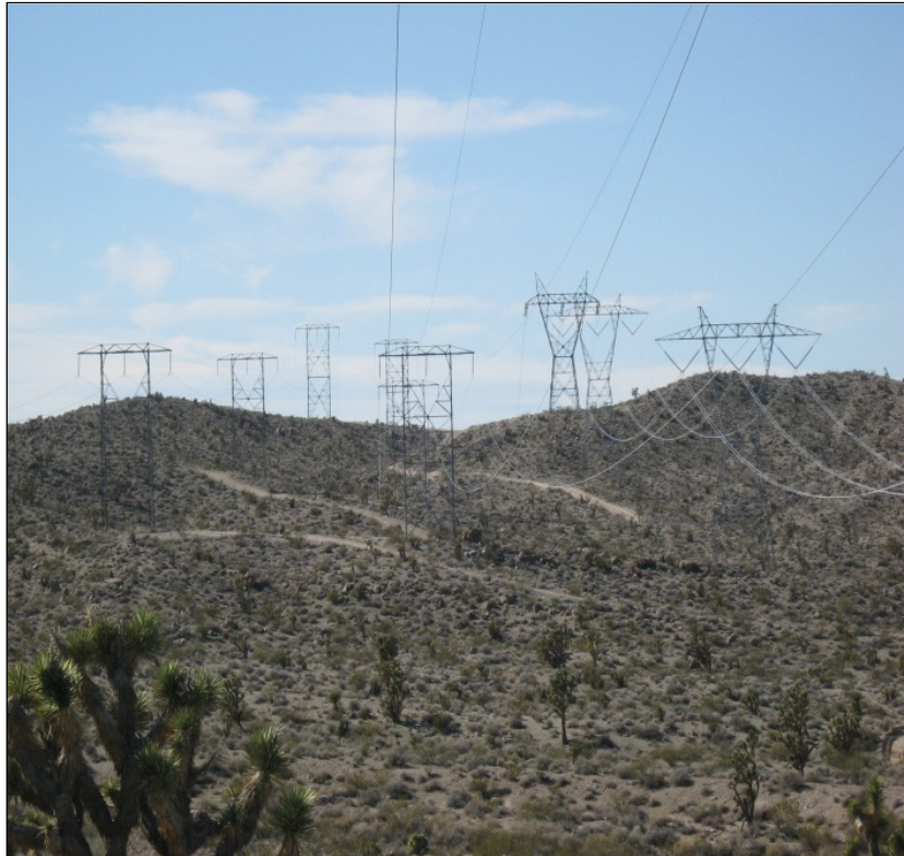
Figure 1. Electrical power lines like these on a linear ROW cross U.S. Government lands to bring power to both rural and urban areas of the Nation. Source: Office of Inspector General (OIG) photo.
