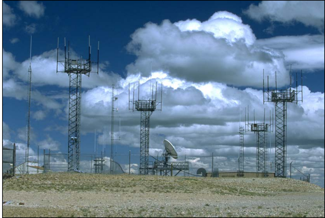
Figure 2. Hundreds of communications sites like this one dot Federal lands. The Department grants companies ROW for their use. Source: BLM photo.
