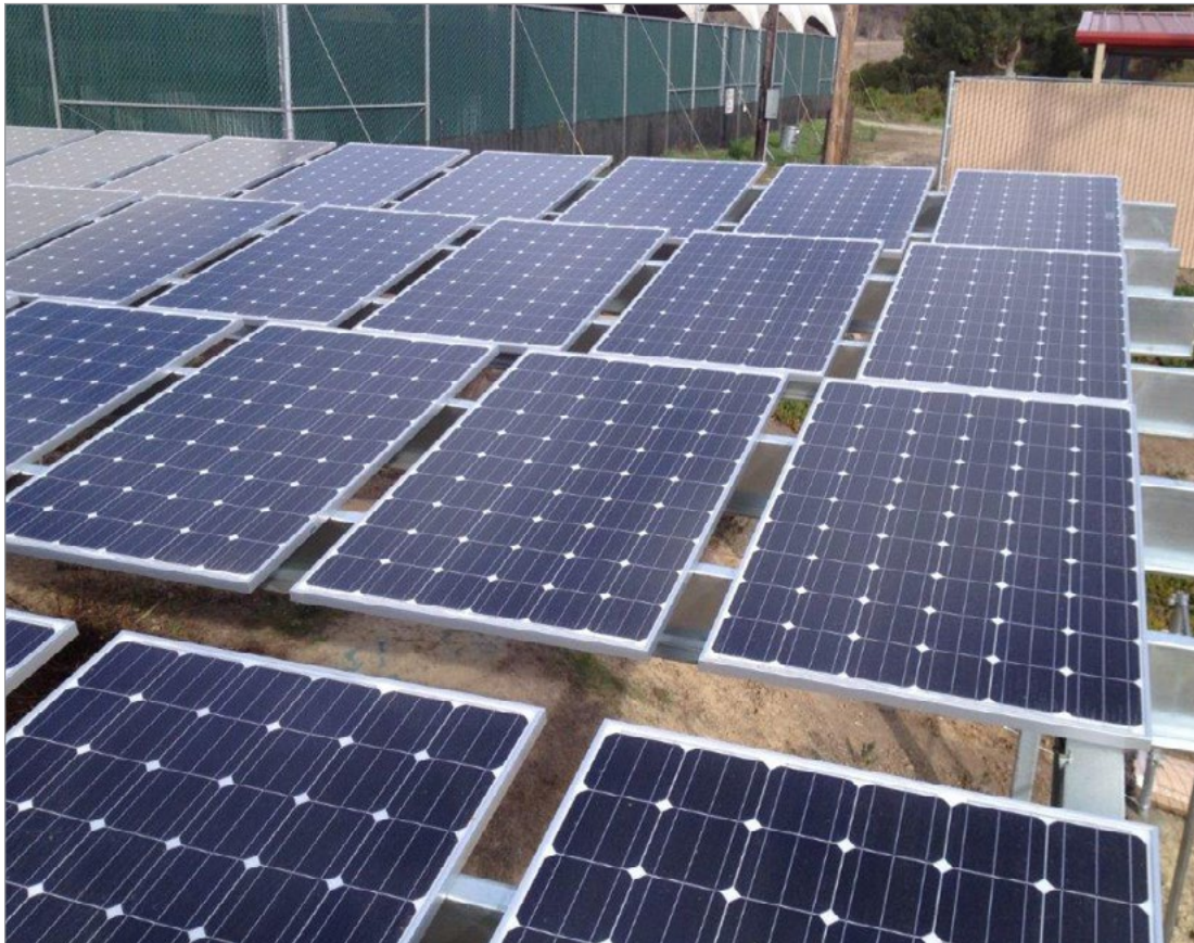
Figure 1. Solar Panel Ground Mounted System Source: MCB Camp Pendleton Energy Office Manager.
