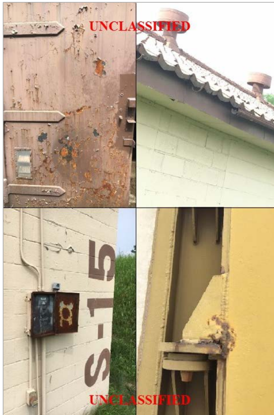
(U) Figure 4. Maintenance Deficiencies Observed: Rusted Door, Missing Gutter, Damaged Door Hinge, Rusted Breaker Box (Clockwise, From Top-Left)
