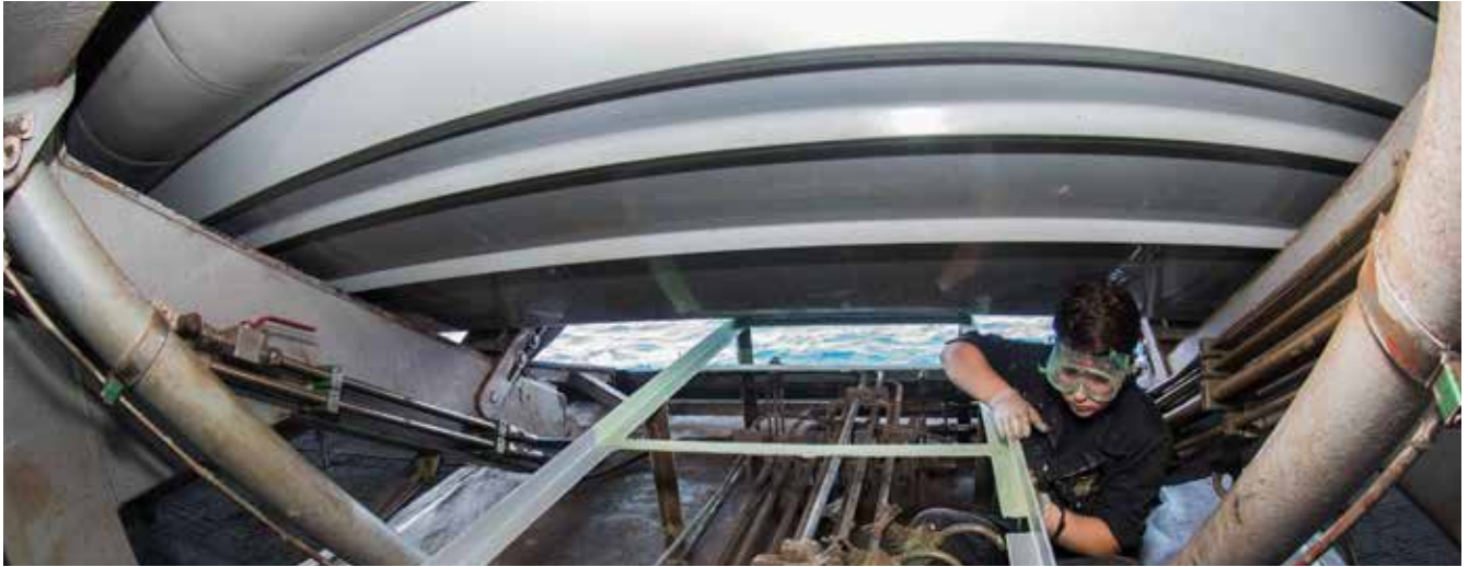
Sanding corrosion off metal on the boat davit. (U.S. Navy photo by Mass Communication Specialist Seaman Apprentice Neo Greene III/Released)
