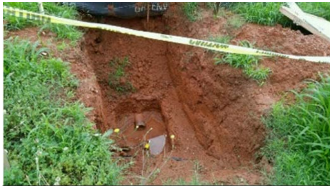
Figure 2 – Capped utilities in front of 211 Bunker St., Spartanburg, SC
