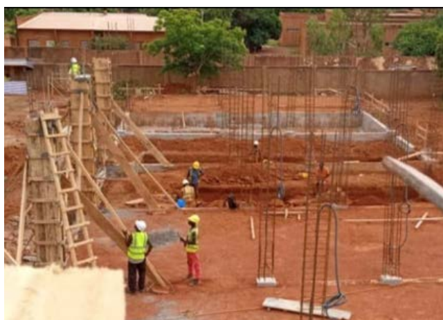
Figure 4: Site view of the construction of facility for the Burkinabe military under the Vehicle Maintenance Facility contract. (SkyBridge photo, August 2019)
