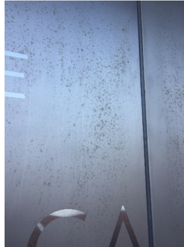
Figure 4: Stainless-steel panels on the front of the new office building at Embassy The Hague.
