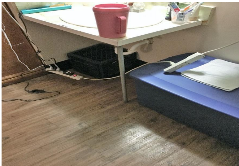
Photograph 13: “Daisy-chained” power strips (one power strip plugged into another power strip).
