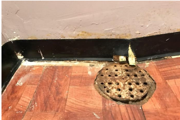
Photograph 13: A rust-covered floor drain and peeling paint in a bathroom (MN).
