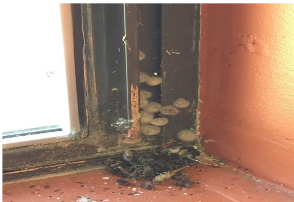
Photograph 17: Facilities were not safe and clean (MS).
