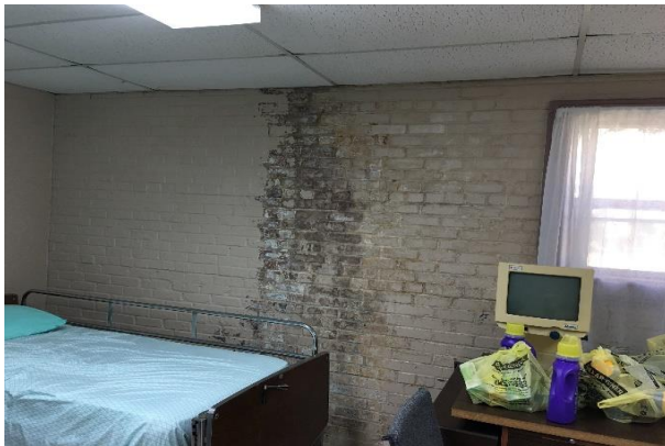
Photograph 1: A bedroom had water damage and mold (MS).
