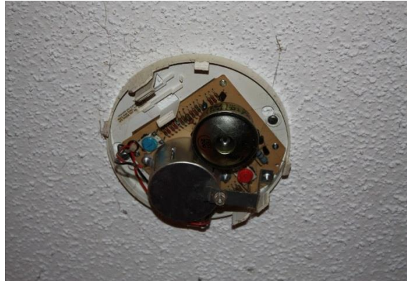
Photograph 8: Smoke detector wiring was uncovered (MN).
