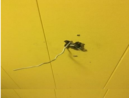
Photograph 7: Electrical wiring was exposed (MS).
