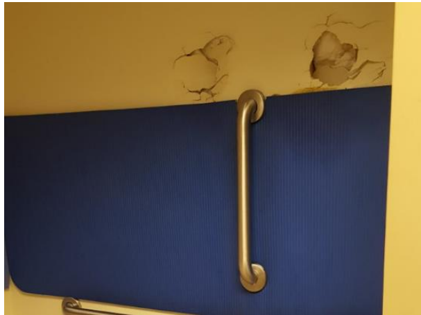
Photograph 15: A wall in a bathroom had holes (WI).
