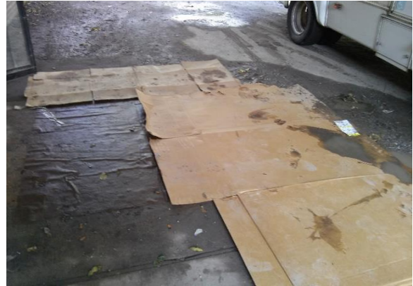
Photograph 14: A participant unloading area was unsafe (MS).
