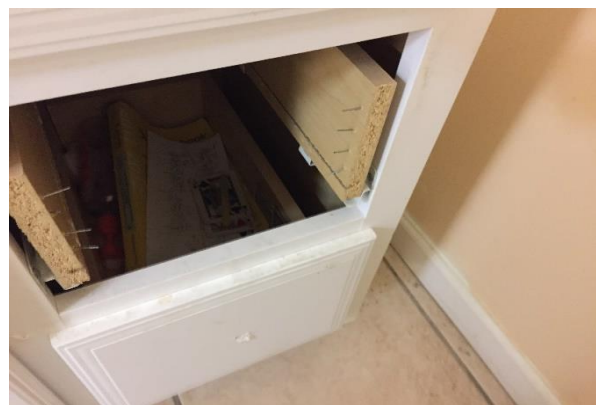
Photograph 18: One area contained exposed nails (MS).
