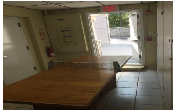
Photograph 12: A game table partially blocked an exit (IL).
